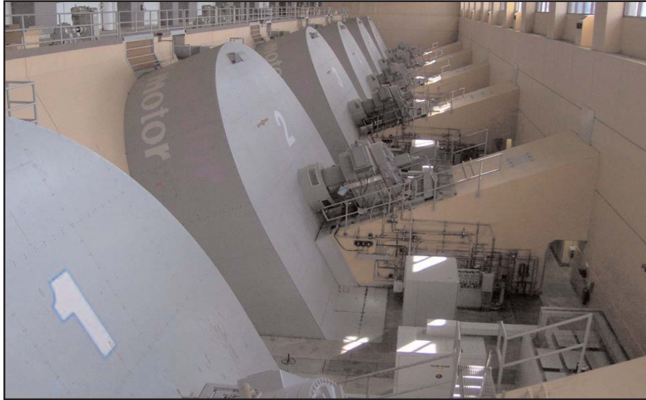
Turbines at the hydroelectric plant at the Harry S. Truman Dam
