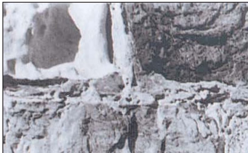
Figure 3. Stone and Mortar Deterioration.
