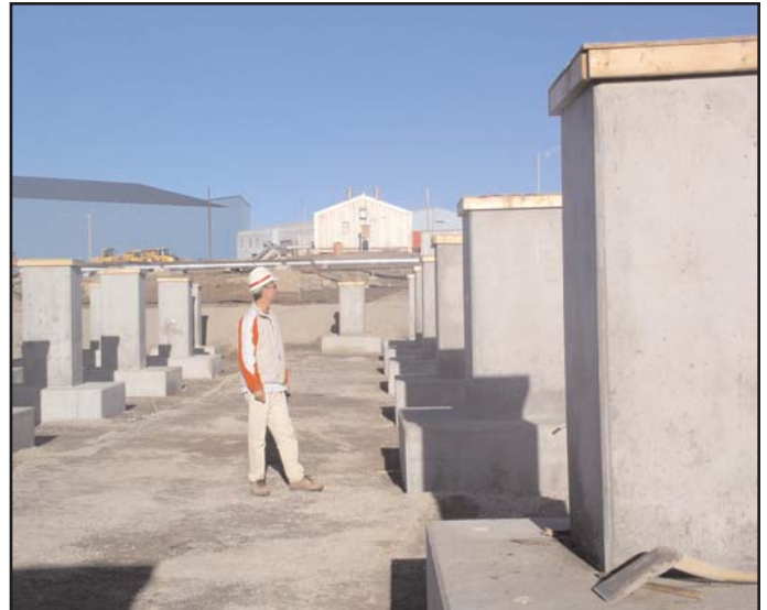
Paul Kara, Lead Engineer, inspects placement of concrete footings, all of which were installed within a 24-hour time period. Credit: Dino Vizzoca, USACE, NYC.
