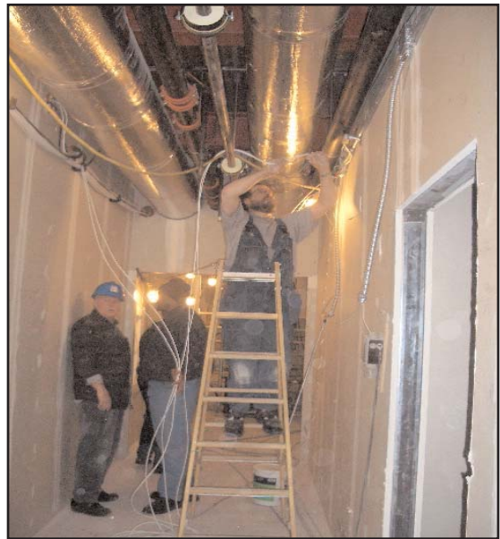
Esben Petersen, MT Hojgaard, discusses the facility's electrical and communication wiring with Sterrett Daniels, Site Engineer, USACE, New York District.
