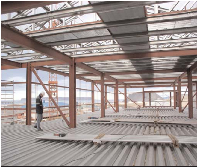
Contractors inspecting installation of flooring system metal decking. Credit: Sterrett Daniels, USACE, NYD.
