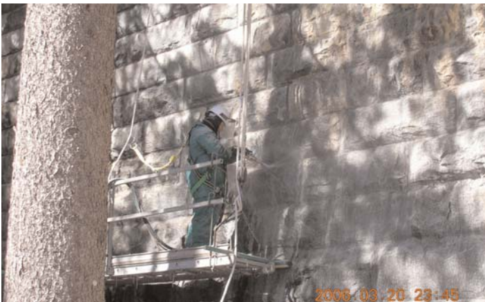
Worker cleans calcite build-up on dam's masonry stones by sandblasting them with small coarse grained silica, glass-like particles, under water pressure (Credit: Milton N. Ricks, Project Engineer, Corps, New York District)
