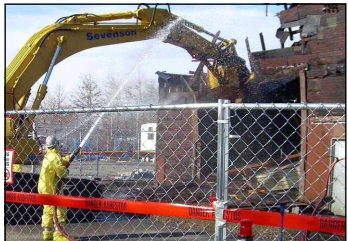
Commencement of building demolition at the Cornell Dubilier Electronics Superfund Site on Feb. 28, 2007
