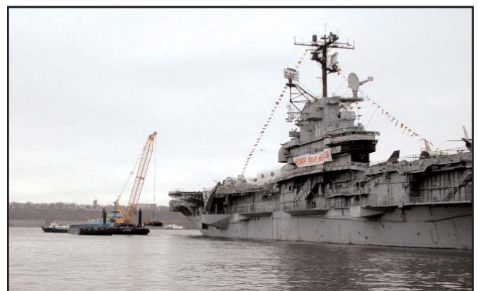
Workers dredge along the aft end of the starboard side of the Intrepid.
