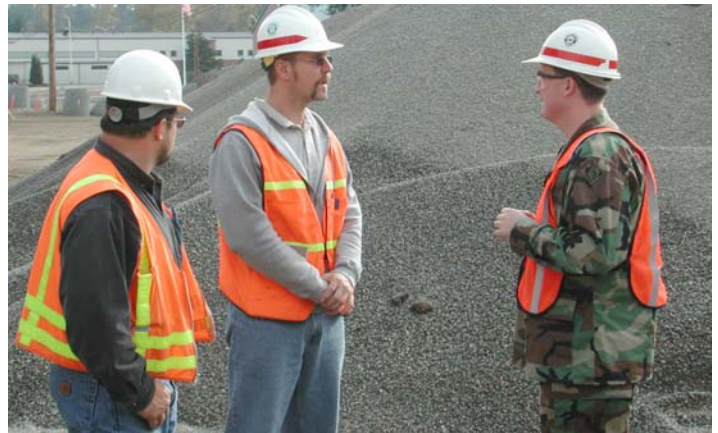
From left, Roger Silva, Roger Kohls and Maj. Steve Ward discuss quality control of materials on the FY02 barracks project.
