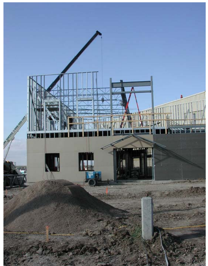
A crane moves beams into position atop the helicopter operations facility at Malmstrom AFB.
