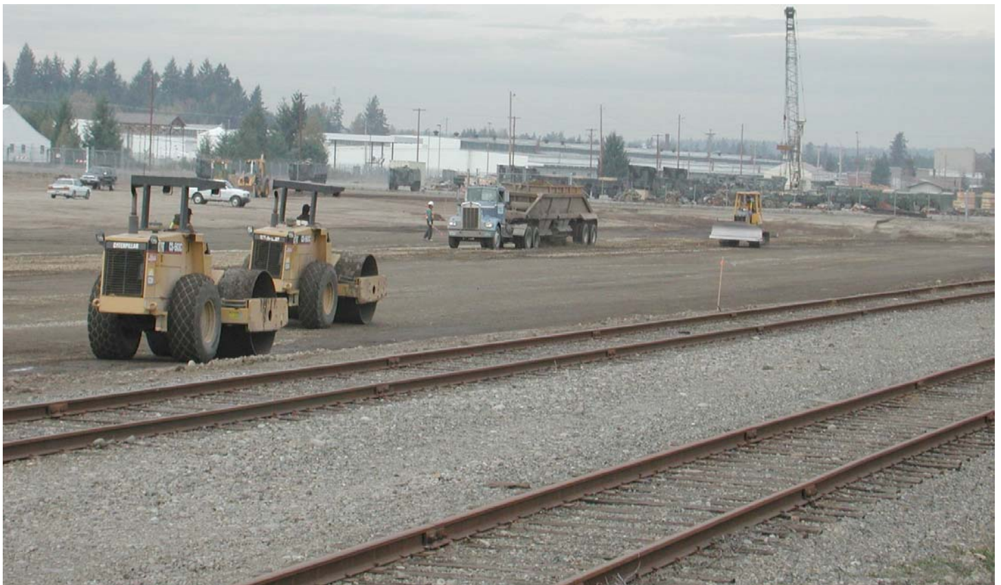
ICON Company completes compaction work on the new rail yard for the Fort Lewis Deployment Facility.
