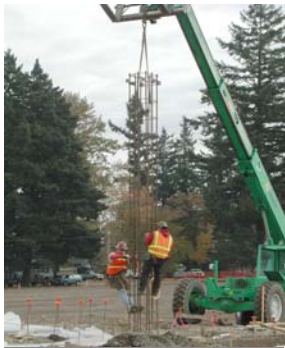
On the cover: Iron workers tie rebar for columns on the Deployment Facility’s “Marv’s Yard” warehouse. Read about immense construction efforts at Fort Lewis and points east.
