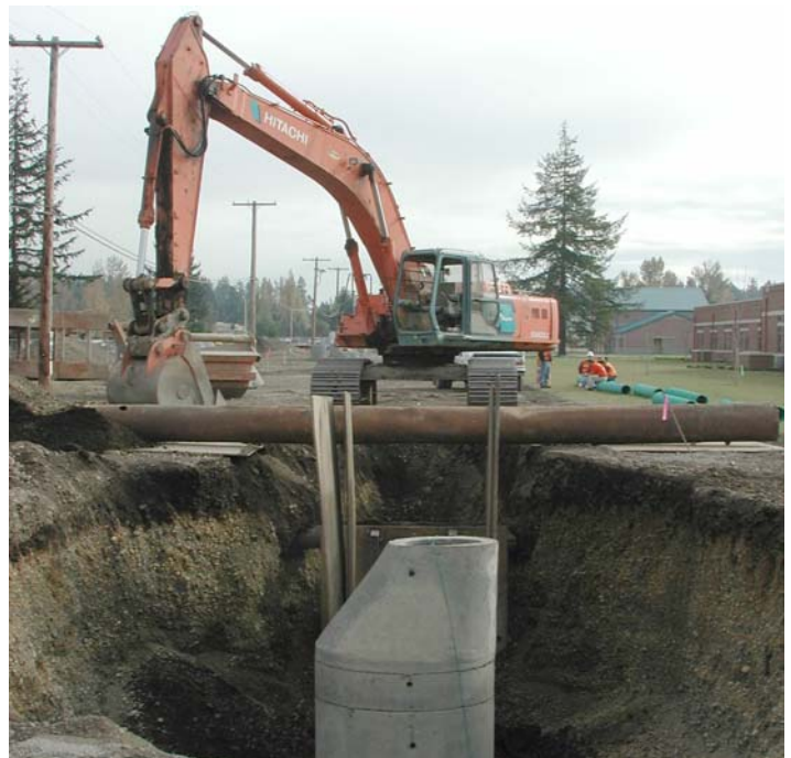
Under the able eyes of Seattle District construction reps, Baugh-Skanska provides new utilities for the FY02 barracks.
