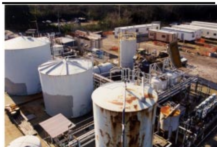
The existing ground water treatment plant will need repairs and upgrades after being damaged by the Nisqually earthquake.
