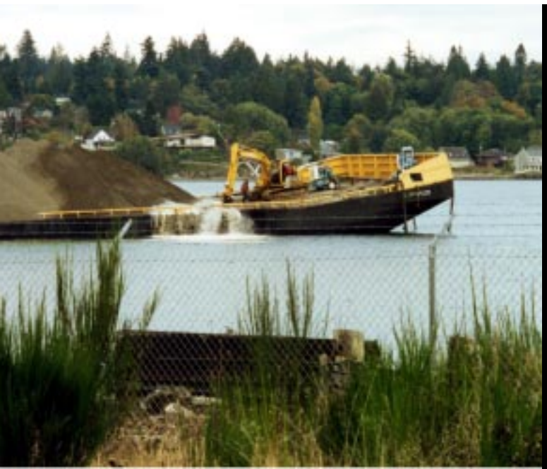
The site shows sheet pile wall installation, excavation of the embankment; above, the wash-off method of cap removal at Eagle Harbor.
