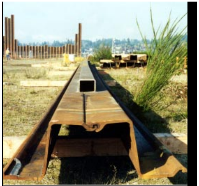
Sheet piling made out of special steel is purchased from a manufacturer in England.
