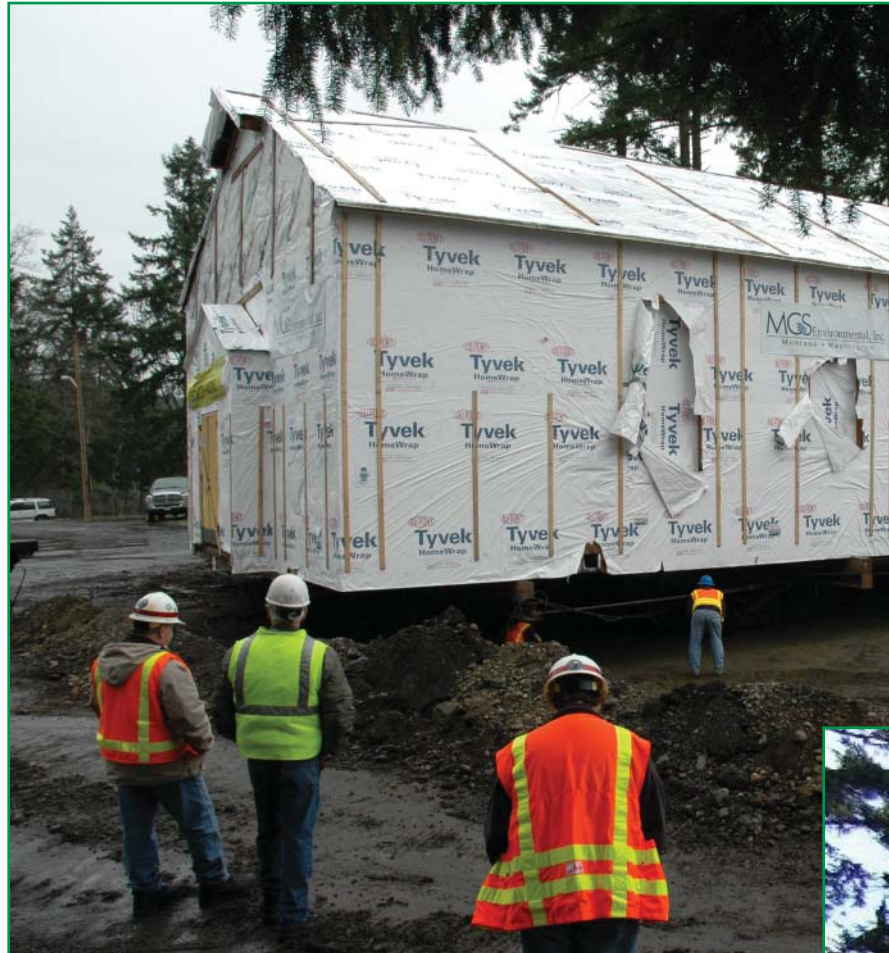
Above: Rich Littooy, Barry Poirrer and Elizabeth Chien observe as the chapel is carefully placed into its new location. Right: With the steeple to its side, the chapel is hoisted up on wheels and is ready for its journey. (Kayla Overton Photos) Below: Final rendering of what the chapel will look like once completed. (Rendering Courtesy of Mike Iacono)
