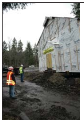
Cover: Seattle District's Elizabeth Chien and Rich Littooy watch along with MSC Environmental Superintendent, Barry Poirrier as a chapel at Fort Lewis is moved to its new location. More photos and story, see pages 6 - 7. (Cover photo by Kayla Overton)
