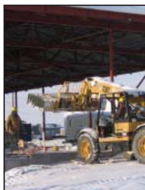
Cover: Workers bundle up against the cold as they off-load construction material at the Corrosion Control Facility, currently being built at Malmstrom Air Force Base, Mont. See more photos and story on pages 6 - 7) (Cover photo by Patricia Graesser)
