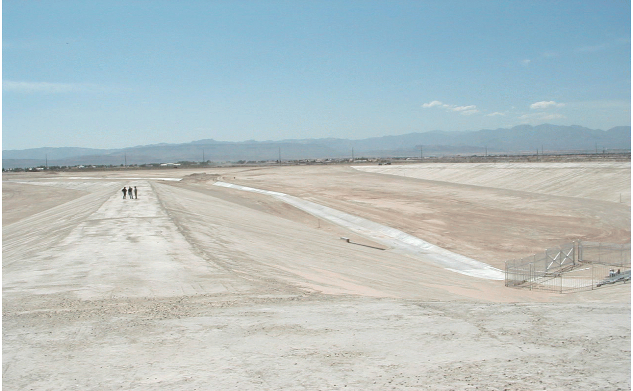
Photo 1. Tropicana Detention Basin . Dike (with individuals atop) separating north and south bays. Outlet works intake structure (with enclosing fence) is at right of photo.
