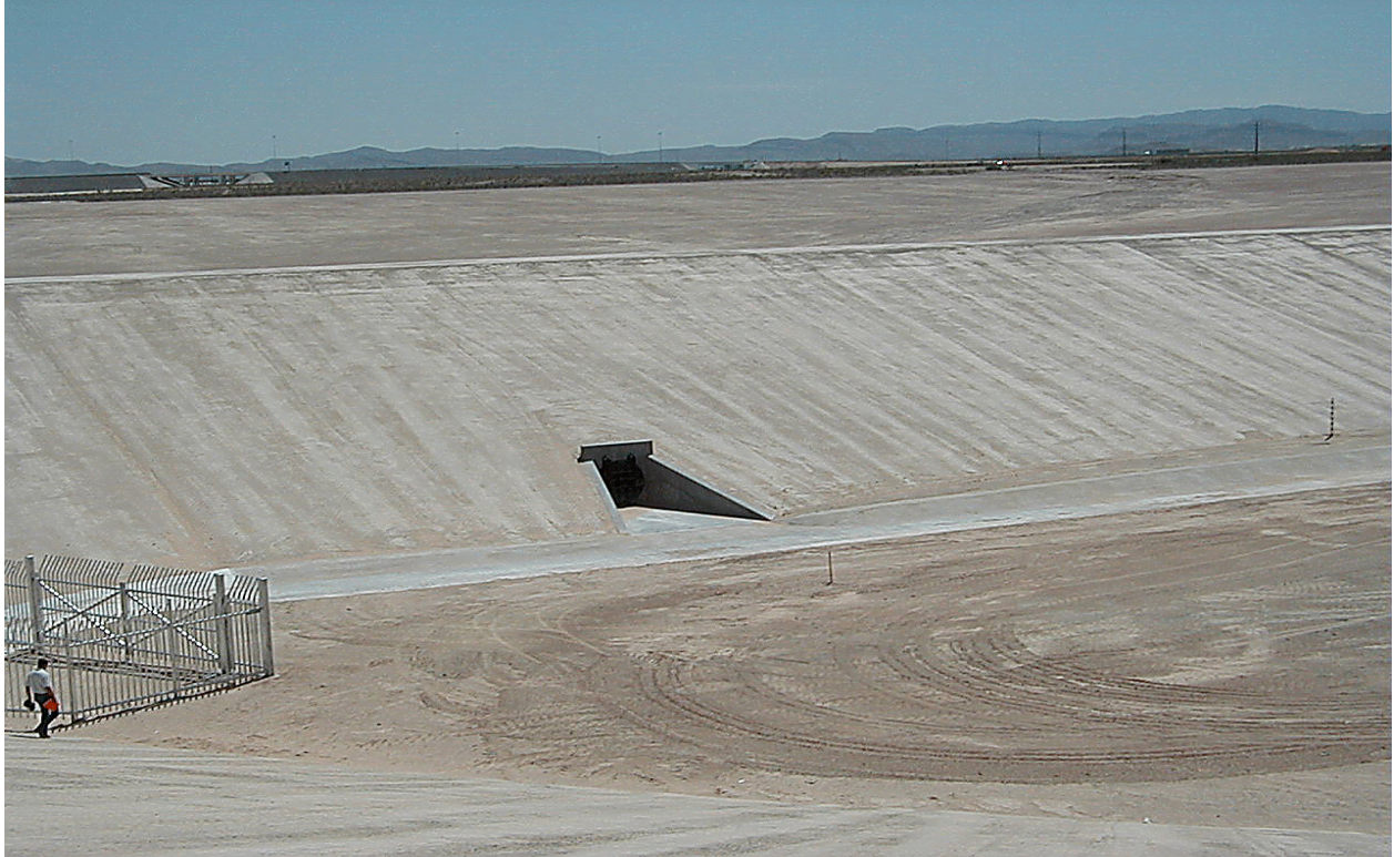
Photo 2. Tropicana Detention Basin . North bay showing downstream end of south-to-north bay conduit.
