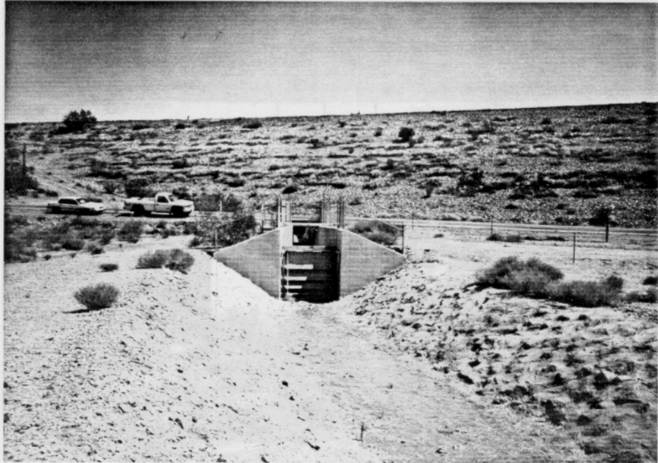
Photo 2-09. Conservation Outlet Works Radial Gate at the Downstream End of the Stilling Basin (view from outlet channel, looking upstream).
