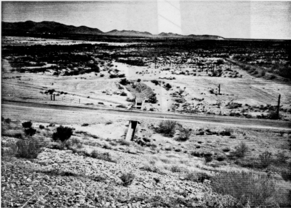
Photo 2-07. Conservation Outlet Works Outlet Channel, Stilling Basin (foreground center), and Vaiva Vo Irrigation Project Canal (left from stilling basin; looking downstream from the main dam embankment).
