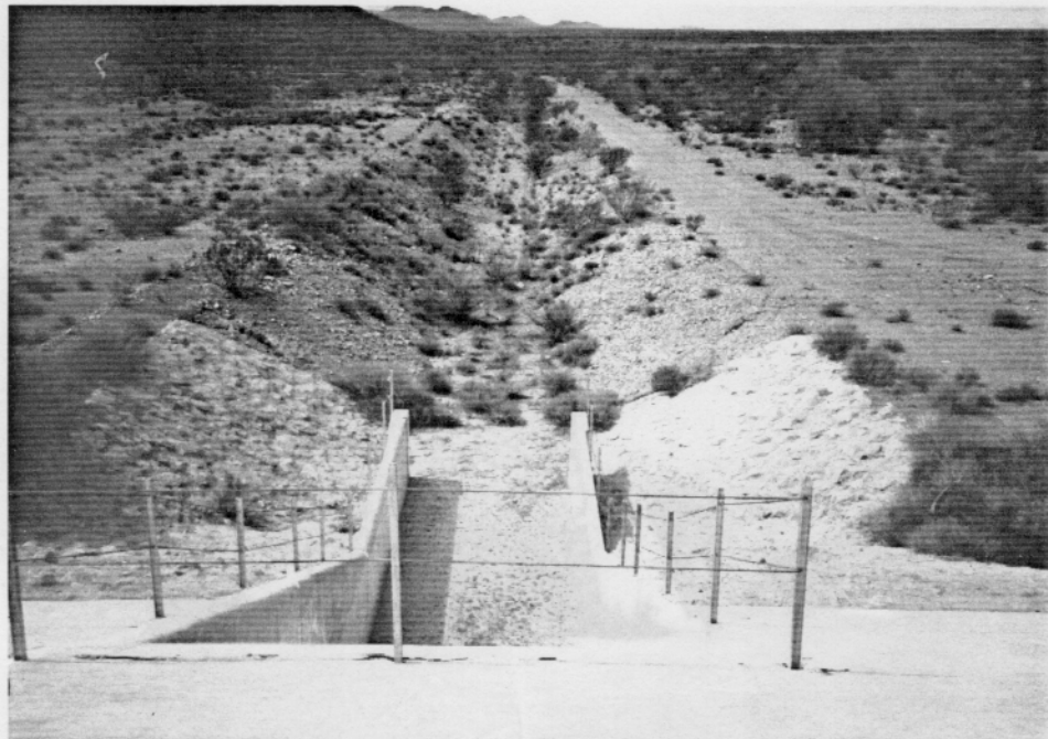
Photo 2-10. Flood Control Outlet Works Approach Channel (view from spillway embankment, looking upstream).
