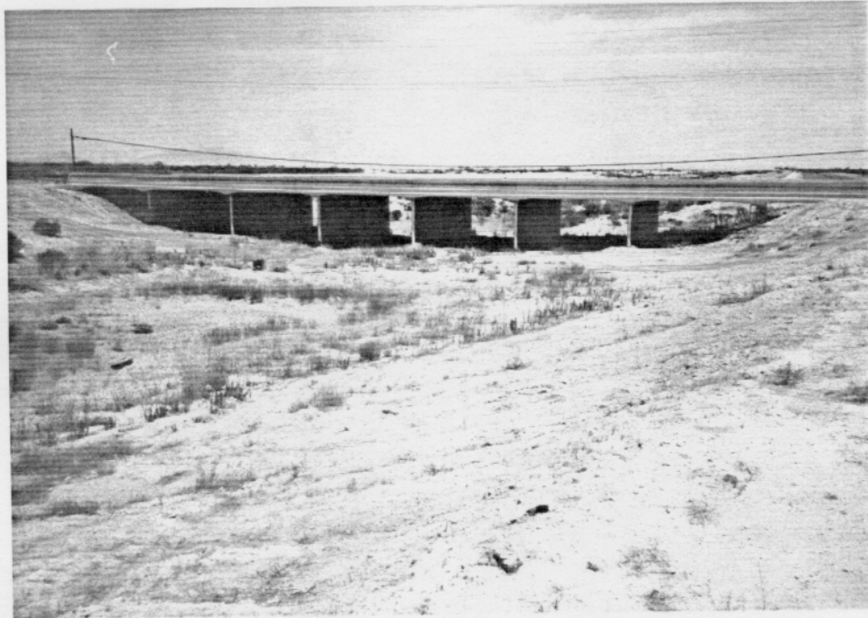
Photo 3-02. Bridge crossing over channelized section of Santa Rosa Wash approximately 17 miles downstream of the dam (looking downstream).
