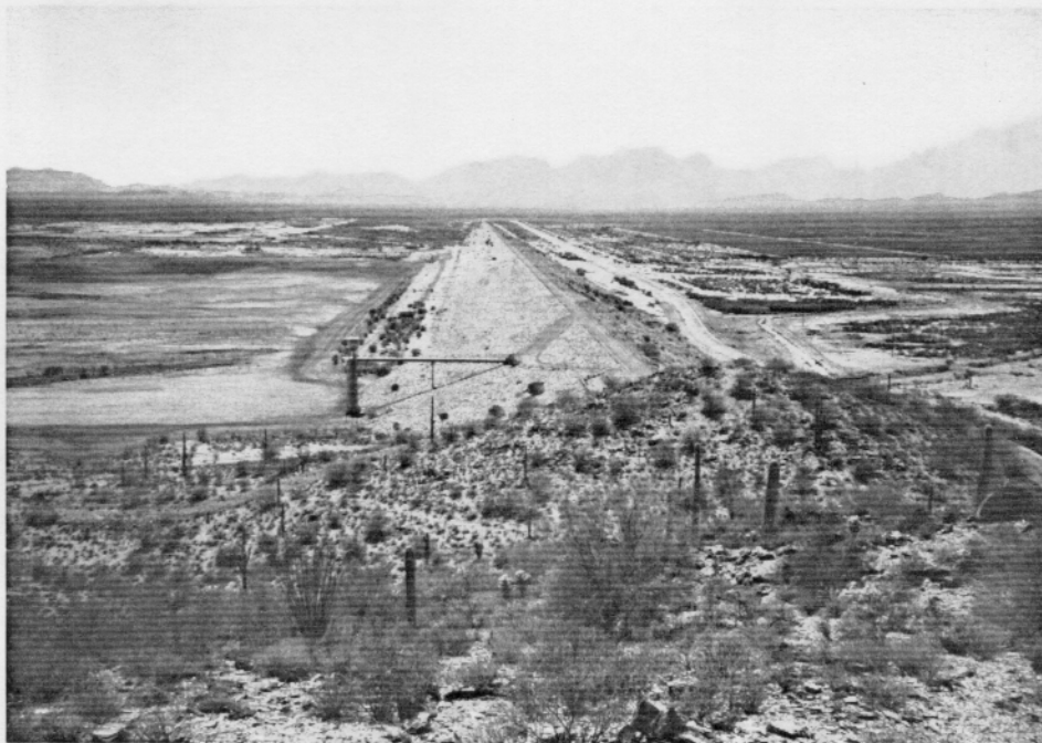
Photo 2-02. Upstream Face of the Tat Momolikot Dam Embankment (looking west from the overlook area).
