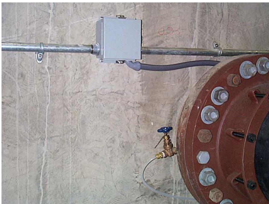
Photo E-3A. Pressure Tap on Cone Valve Pipe
