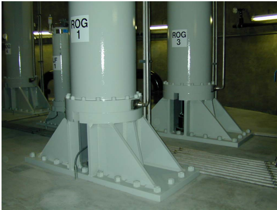
Photo 2-4. RO and LF Gates - Hydraulic Cylinders Inside the Gate Chamber
