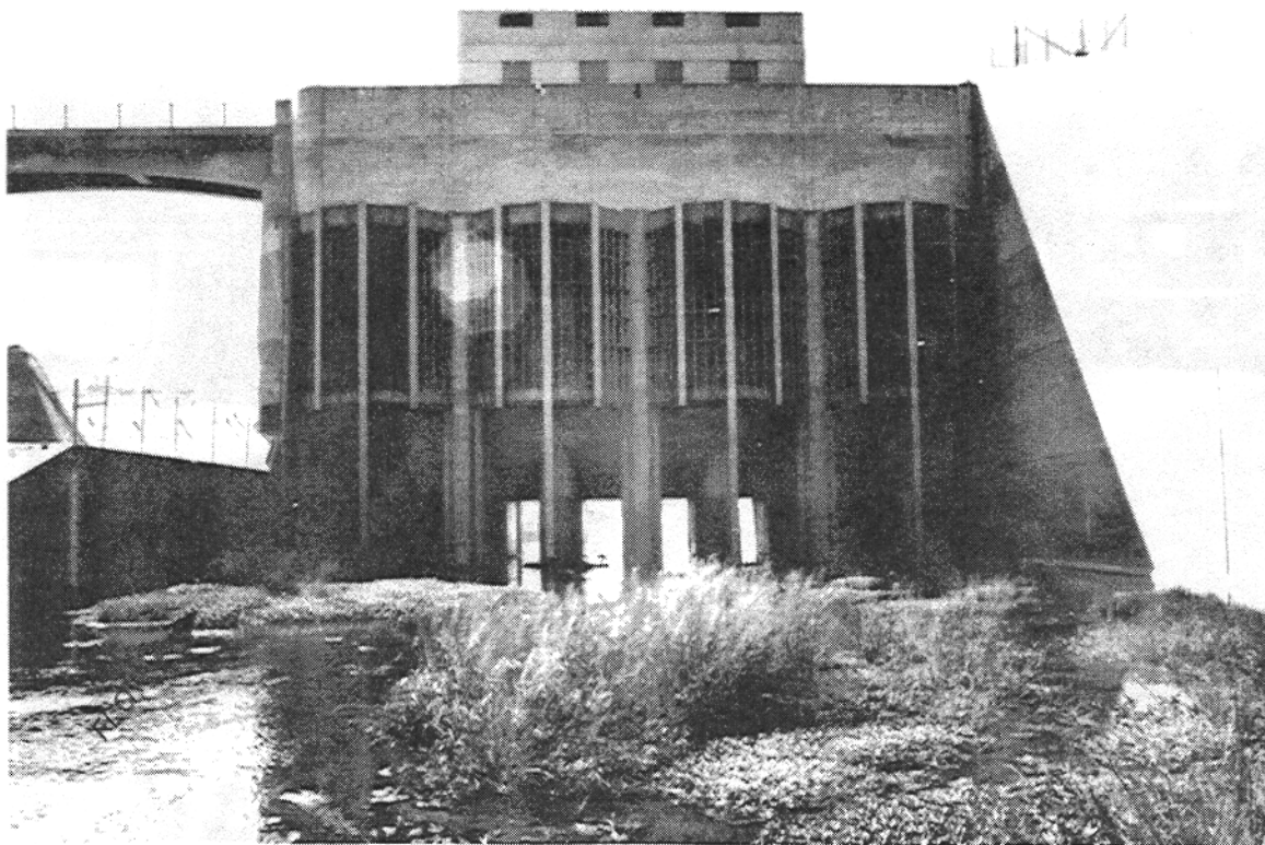
Photo No. 2-13. Outlet Works (gates fully open), with edge of spillway to left (view from channel upstream).
