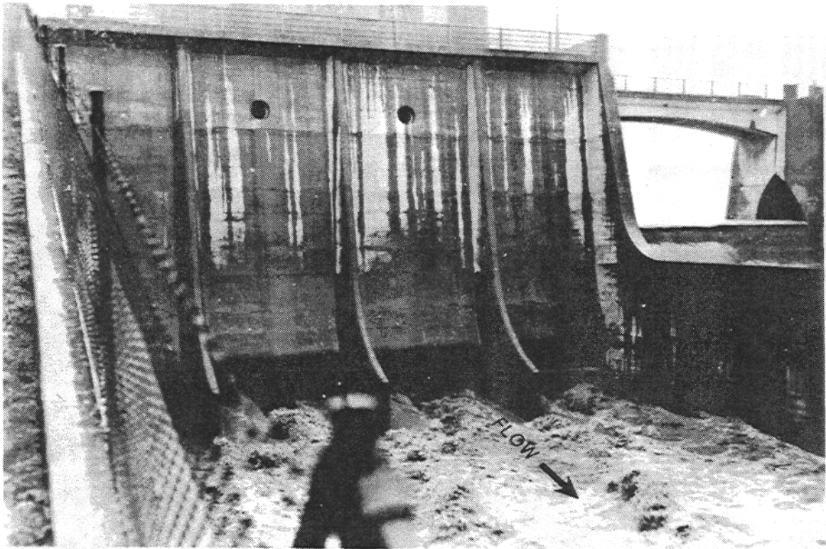
Photo No. 2-16. Outlet Works (all gates open), with edge of Spillway to right (view from alongside channel downstream).
