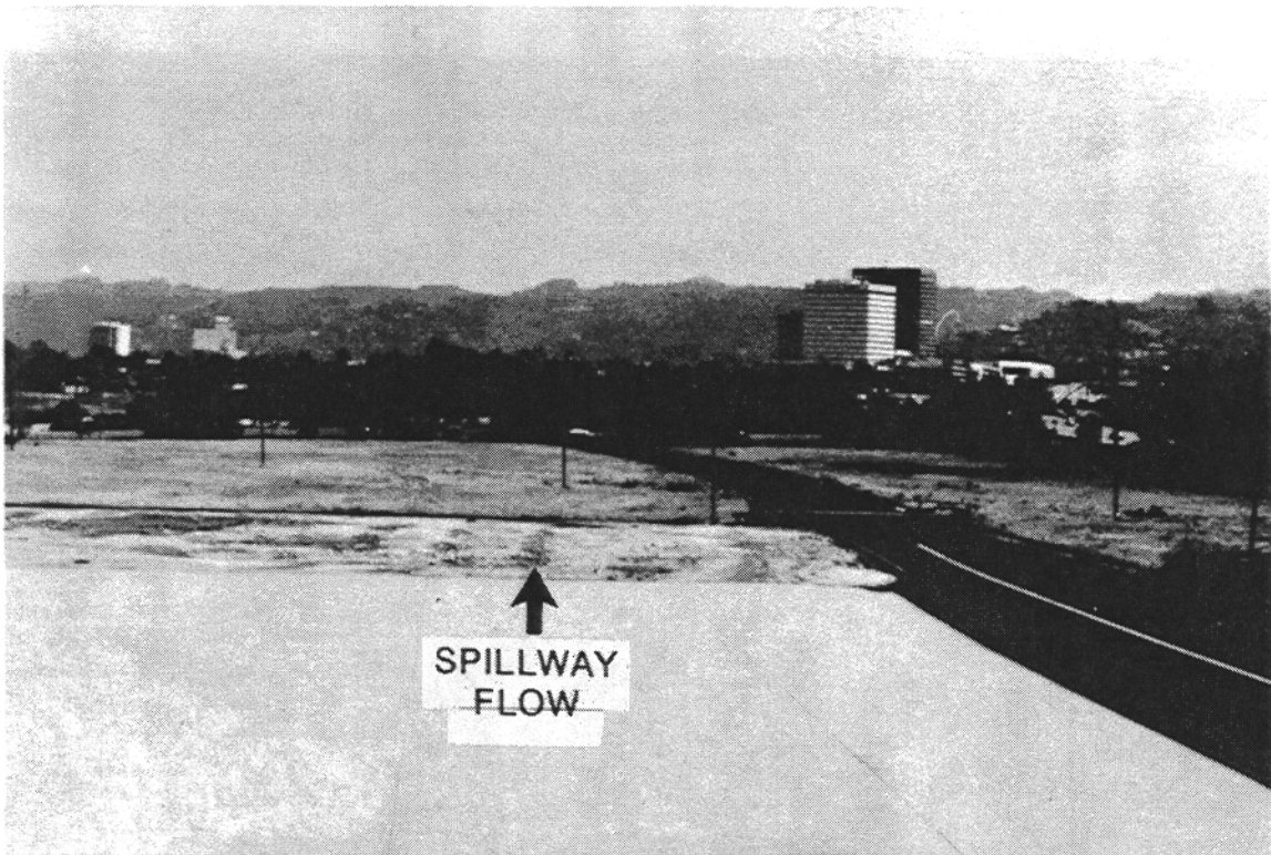
Photo No. 2-23. Spillway Apron, with Outlet Channel to right (view from spillway bridge, toward downstream).
