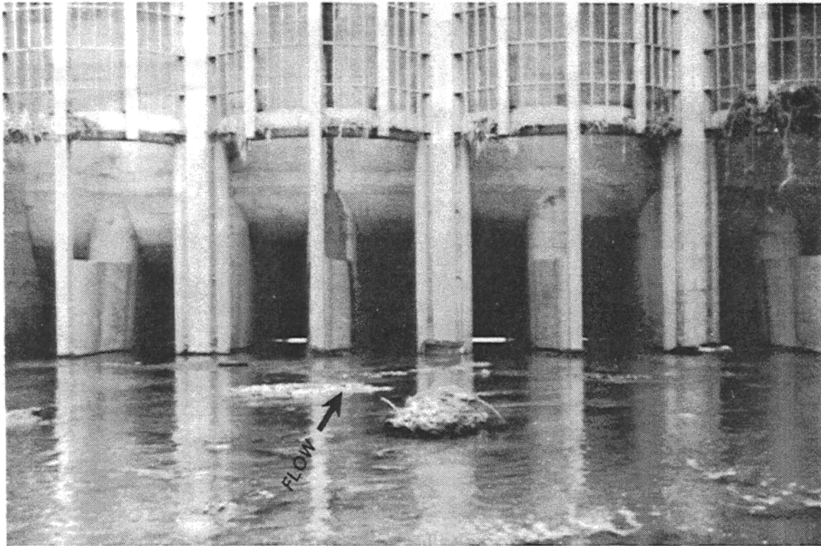
Photo No. 2-14. Approach to Outlet Works (gates partially open) (view from channel upstream).
