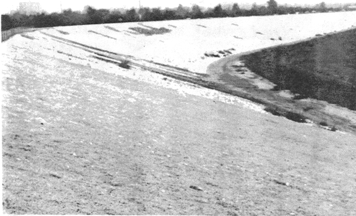
Photo No. 2-09. Upstream Slope of Dam Northeast of Spillway (view toward south, from east embankment of dam.)
