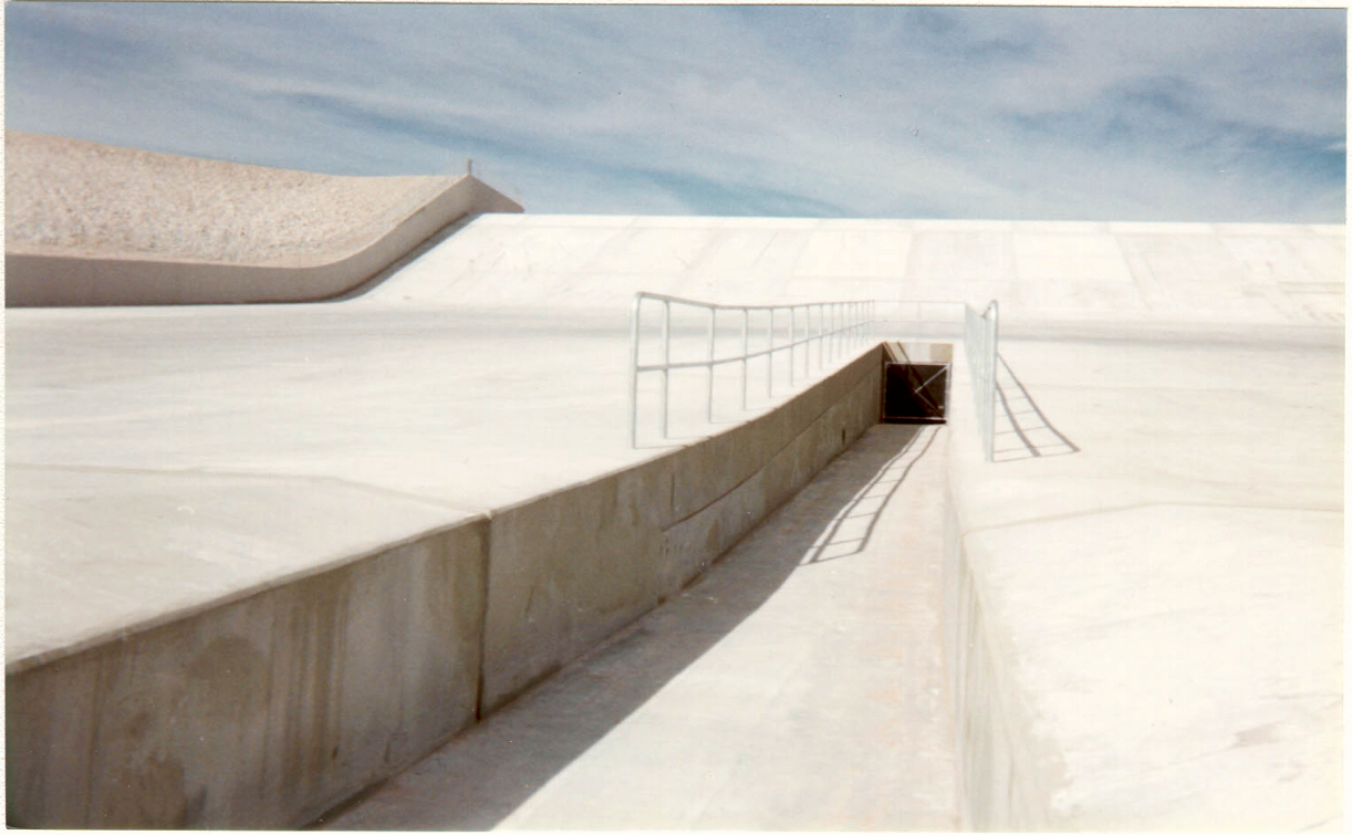
Photo 1. Red Rock Detention Basin . Downstream end of outlet works and auxiliary spillway.
