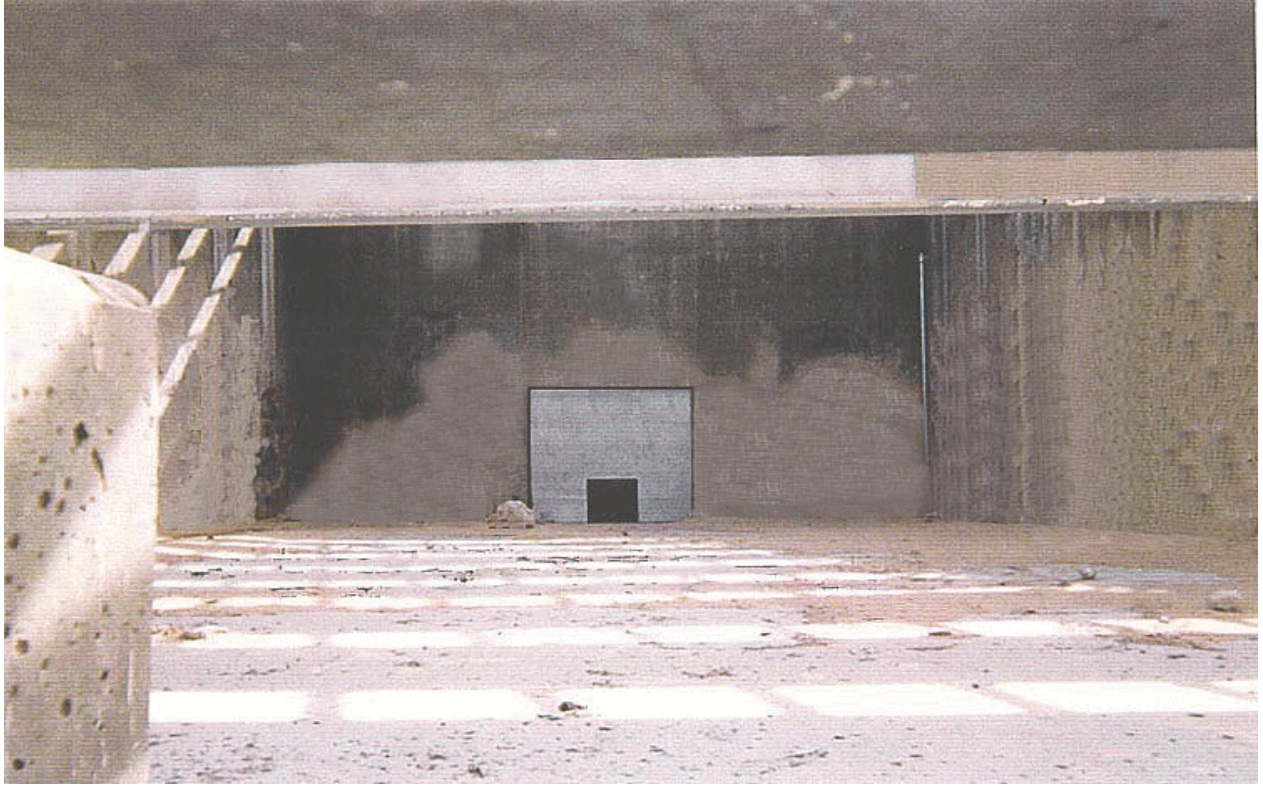
Photo 2. Red Rock Detention Basin . Upstream end of outlet works, showing intake structure constrictor plate.
