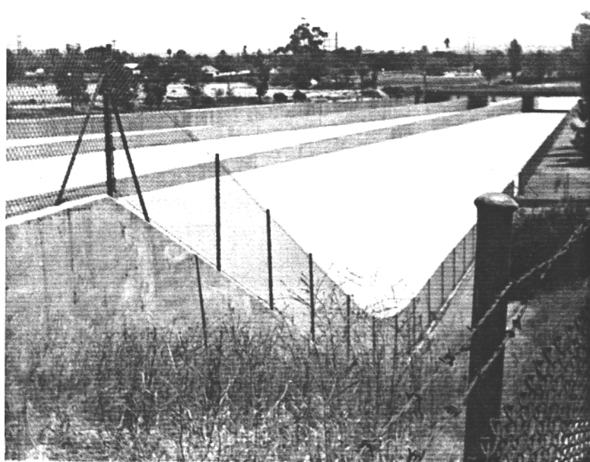
Figure 14. East Branch Lytle Creek Channel Looking SE. The 58,000 c.f.s. Capacity Channel Is 400 Feet Wide With Training Walls At 132 Foot Intervals.
