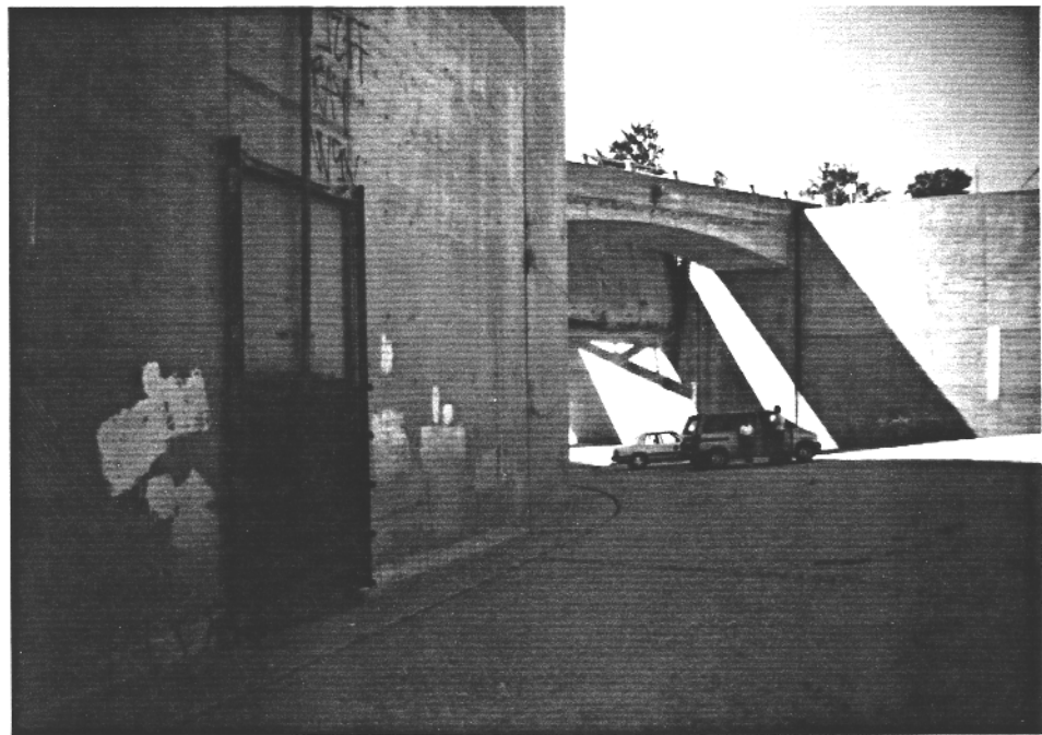
Figure 6. West Branch Lytle Creek Channel Looking SW At Tainter Gate During Gate Test. Unused Bypass To East Branch Of Lytle Creek In Foreground; No Longer Used After Construction Of The East Branch Lytle Creek Channel.
