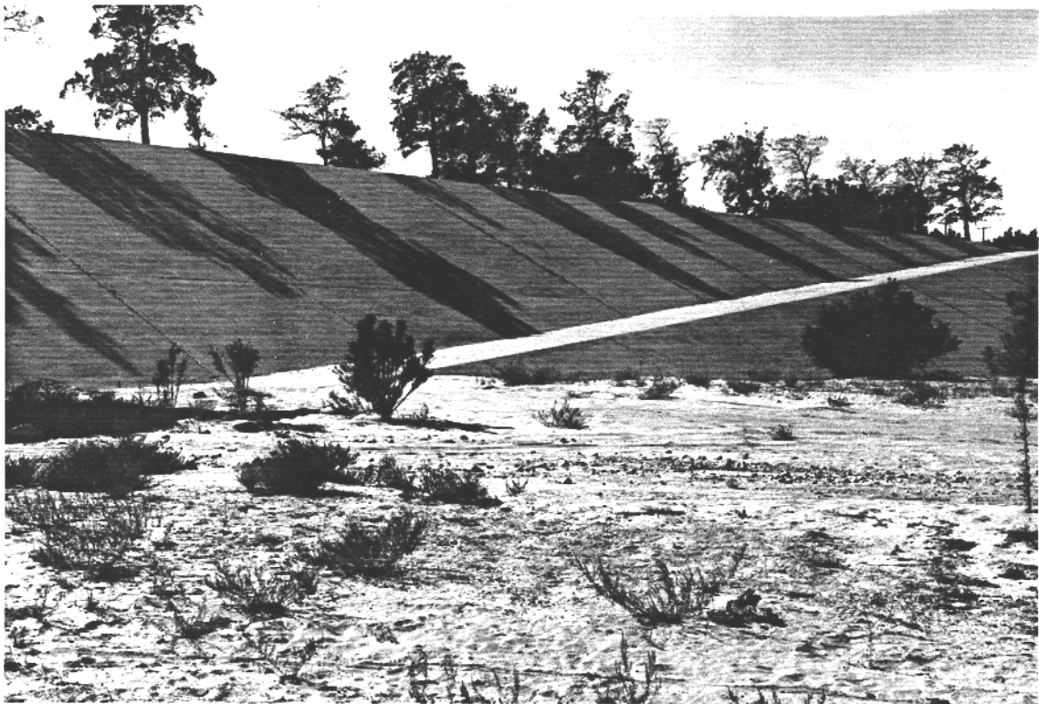
Figure 10. Lytle Creek Intake Structure Looking SW From Intake To West Branch Channel At The West Wing Levee, 1,000 Ft. Long.
