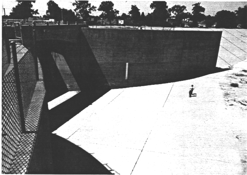
Figure 4. Lytle Creek Intake Structure. West Branch Intake With Tainter Gate Housing. Looking SW With West Wing Levee Beyond Intake.
