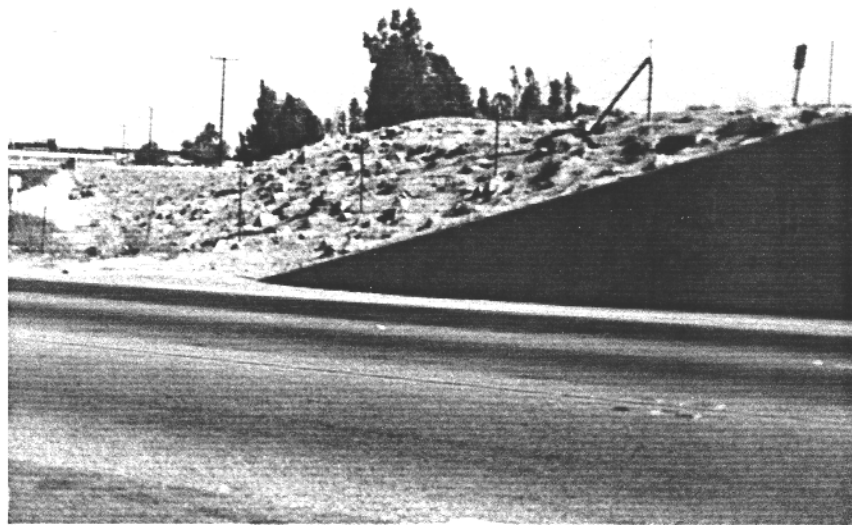
Figure 26. Grouted Quarry Stone Of Island Levee At Highland Avenue Looking South On Lytle-Cajon Drainage, San Bernardino County, California.
