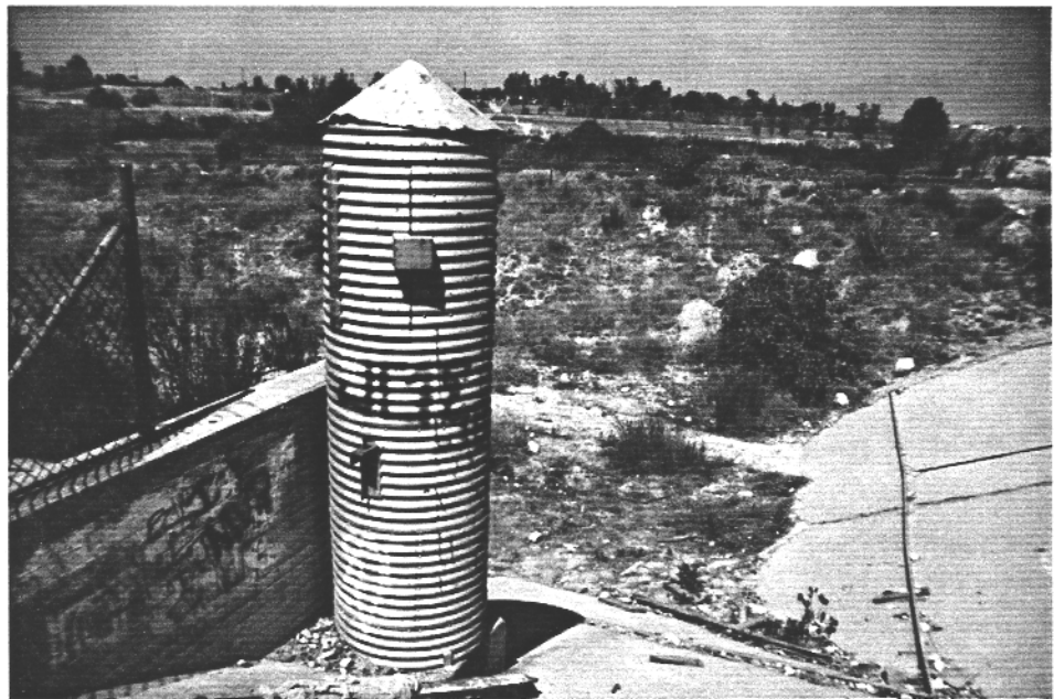
Figure 20. East Junction Of Lytle Creek Intake Structure With Muscoy Levee At Edge Of Original Bypass Spillway. Looking NW, Showing Original Stage Recorder For Spillway. Gauge Is No Longer Used.
