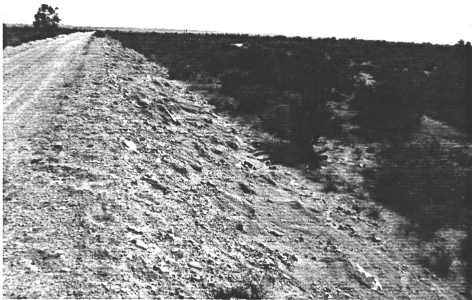
Figure 24. Levee Road On Muscoy Groin No.3 Looking South (Downstream) At Grouted Quarry Stone With Cajon Creek Channel On Right.
