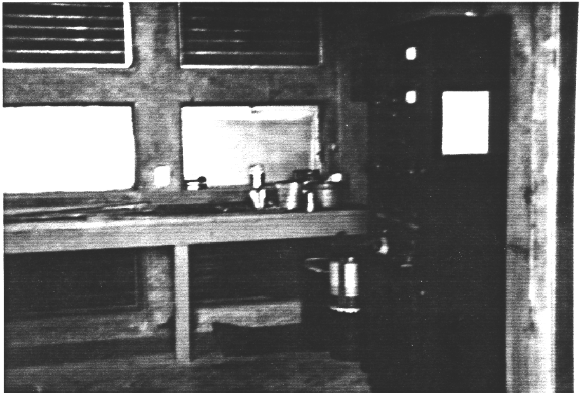
Figure C-1 Interior Of Lytle Creek Intake Control House Showing Electrical Panel For Commercial Power To Operate Tainter Gate.
