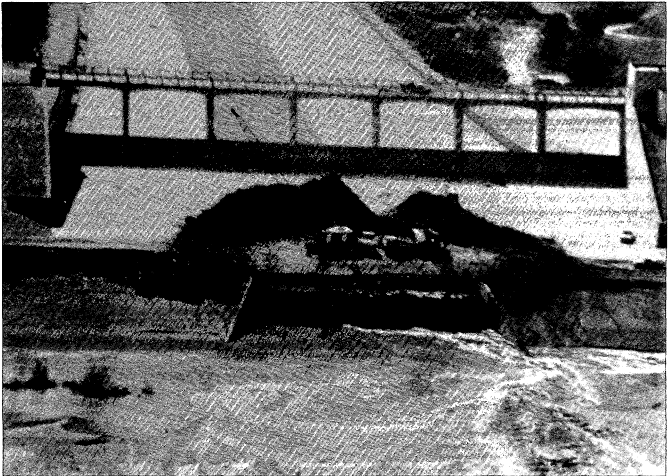
Figure 3-4. Debris at Hansen Dam after March 1, 1983 storm.
