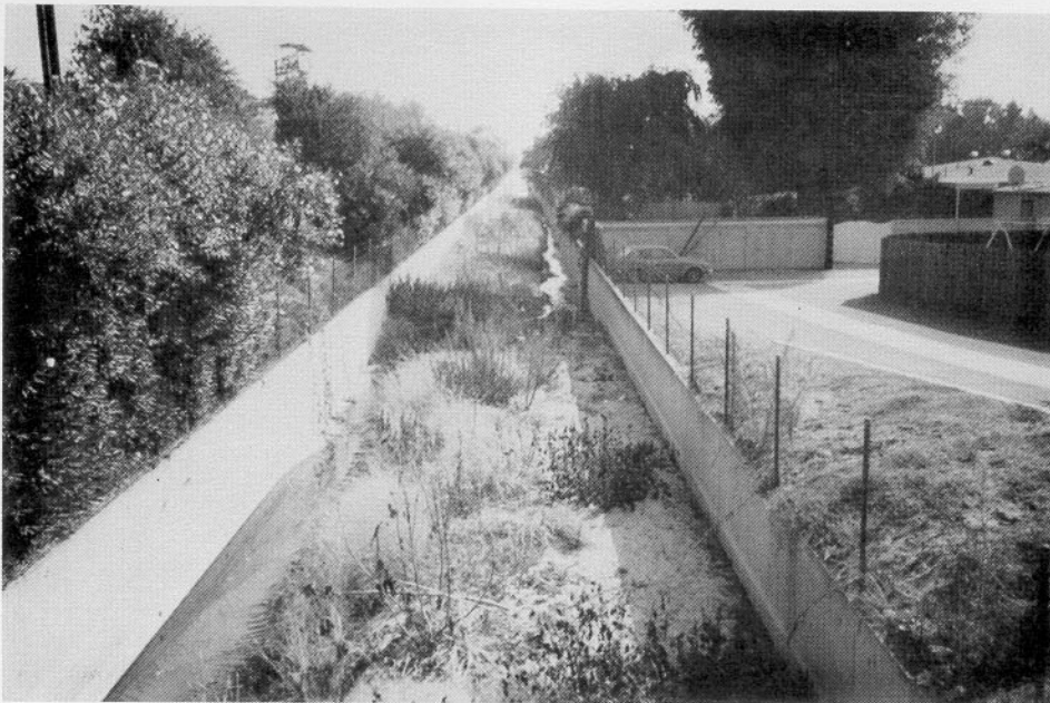
Photo 3-02. Sediment deposition at Basque Avenue (view toward upstream).
