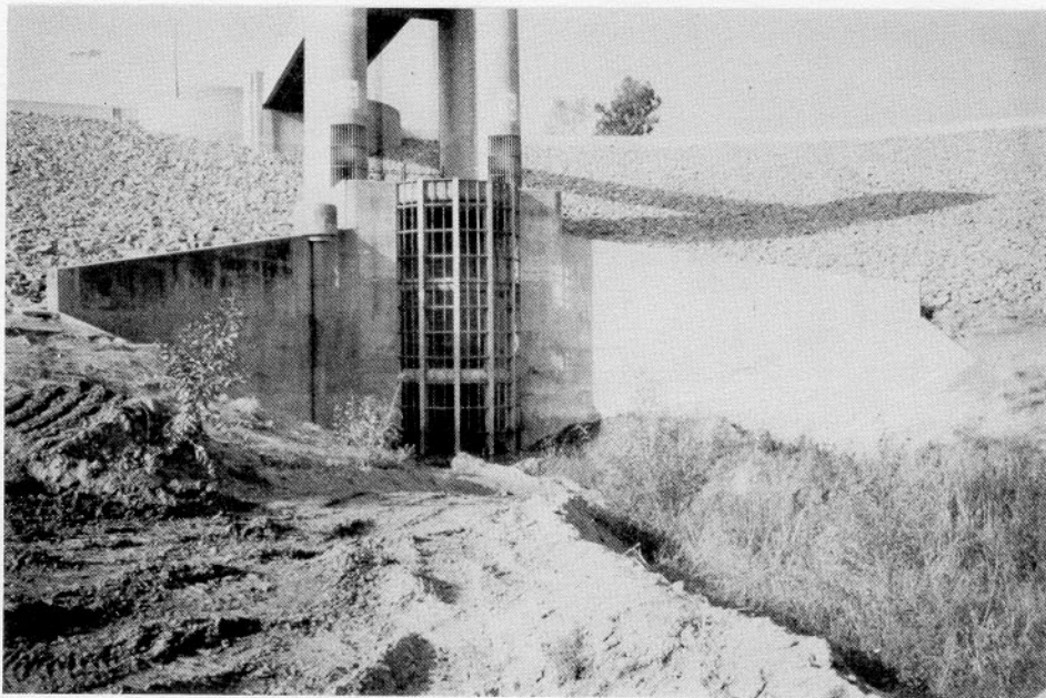
Photo No. 2-04. Outlet works: approach channel and trash rack (view toward downstream).
