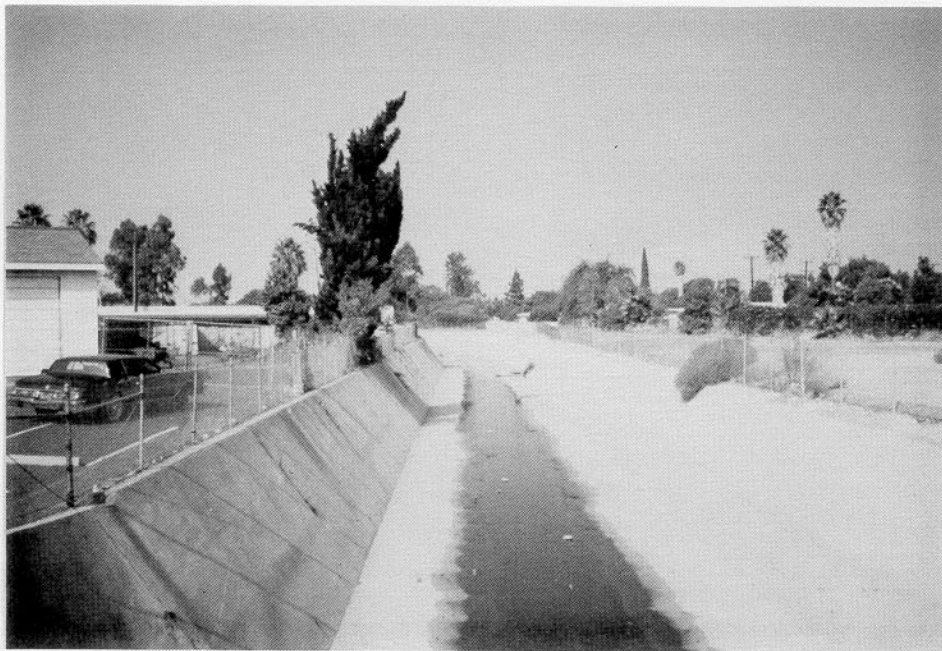
Photo No. 4-04. Trapezoidal concrete channel with 4,900 cfs capacity (view toward downstream from Beach Boulevard).
