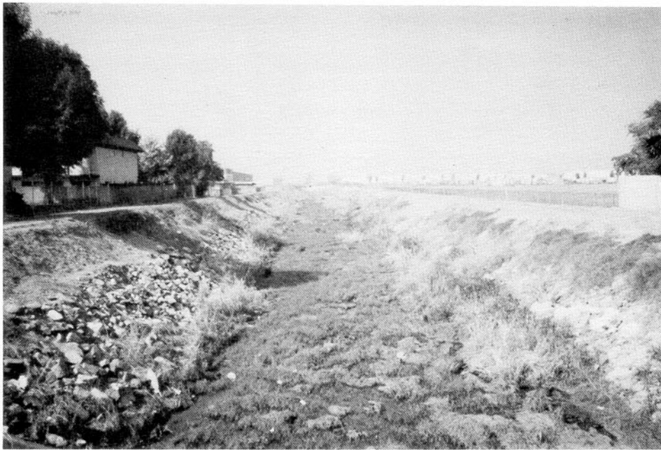
Photo No. 4-05. An unlined channel with 4,000 cfs capacity (view toward downstream from Western Avenue). Confluence with Coyote Creek is in far background.
