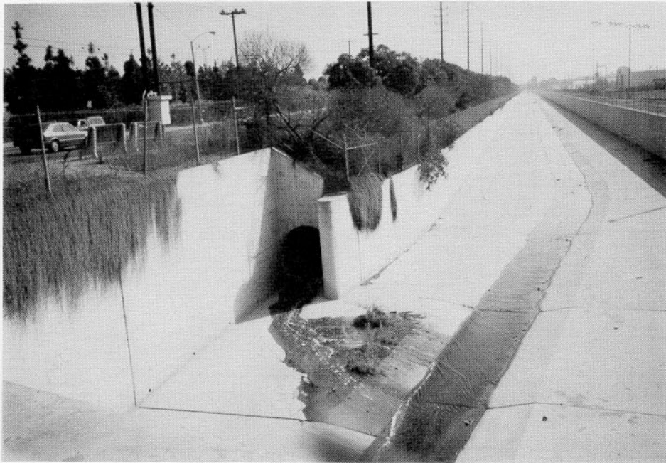
Photo No. 4-03. Rectangular concrete channel with 11,000 cfs capacity (view toward upstream from Gilbert Street).
