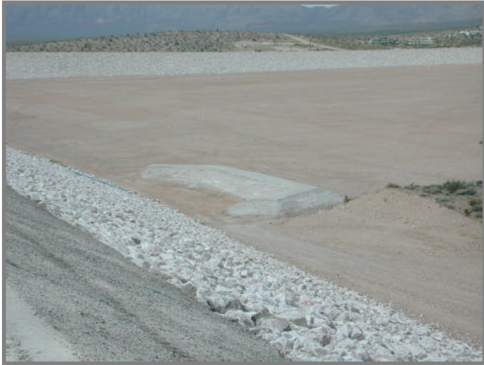
Photo 3. Blue Diamond Detention Basin . Sediment berm.
