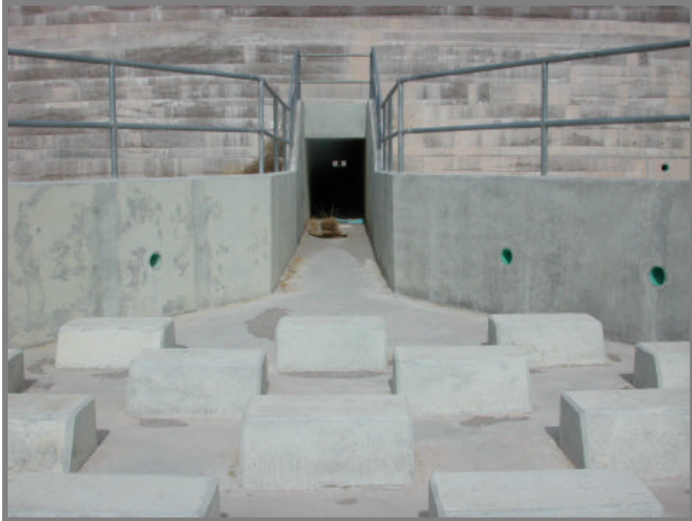
Photo 6. Blue Diamond Detention Basin . Downstream end of outlet works and dissipator blocks.
