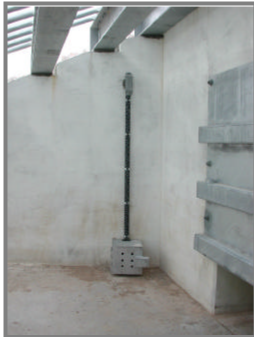
Photo 13. Blue Diamond Detention Basin . Water surface sensor.
