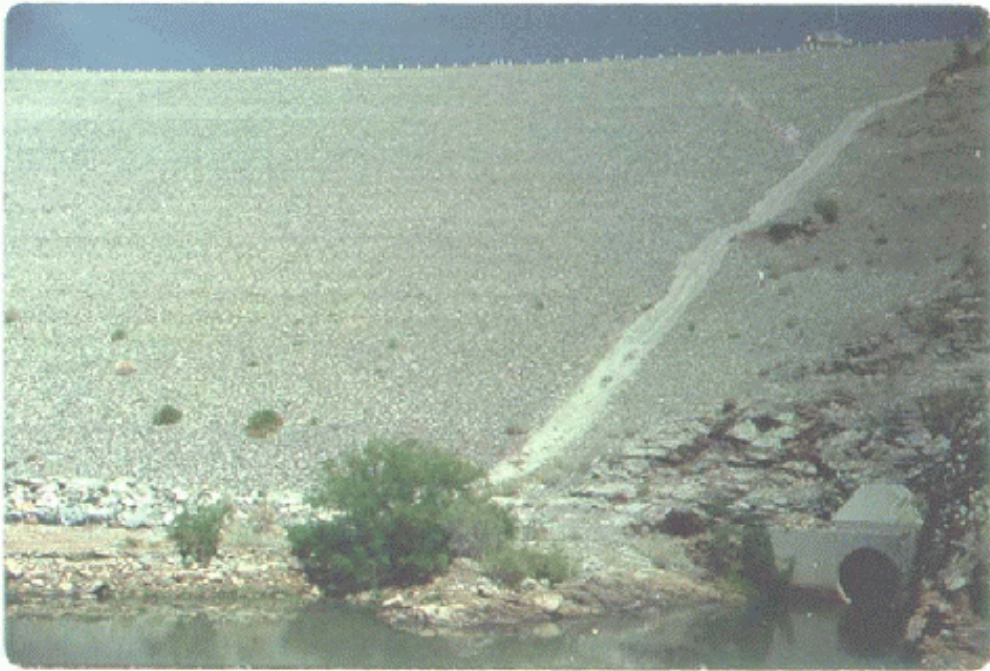
Photo 2-01. Downstream face of Alamo Dam. Outlet works tunnel is in lower right hand corner.
