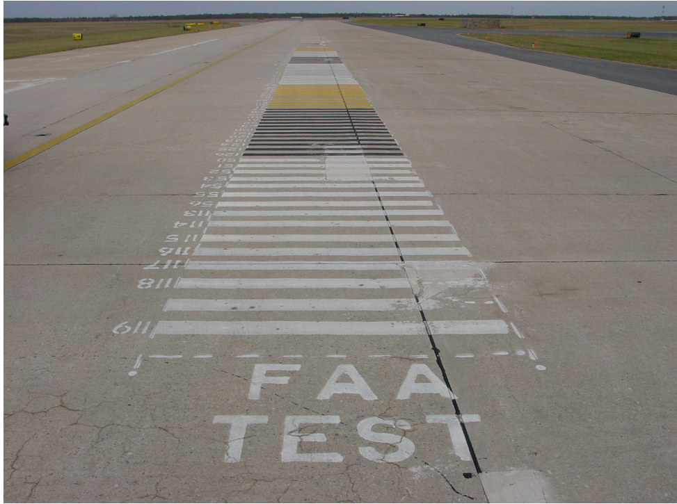
FIGURE 6. LINES AT TAXIWAY HOTEL ON PORTLAND CEMENT CONCRETE
