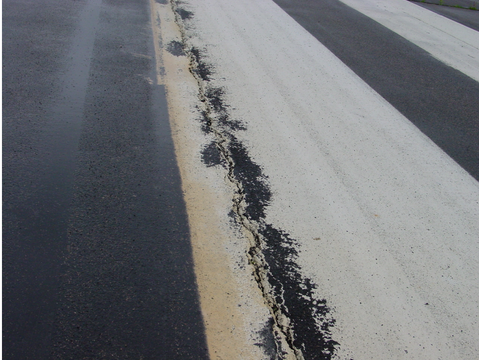
FIGURE 10. YELLOWING OF THE WHITE PAINT AT NEW BEDFORD AIRPORT, NEW BEDFORD, MASSACHUSETTS
