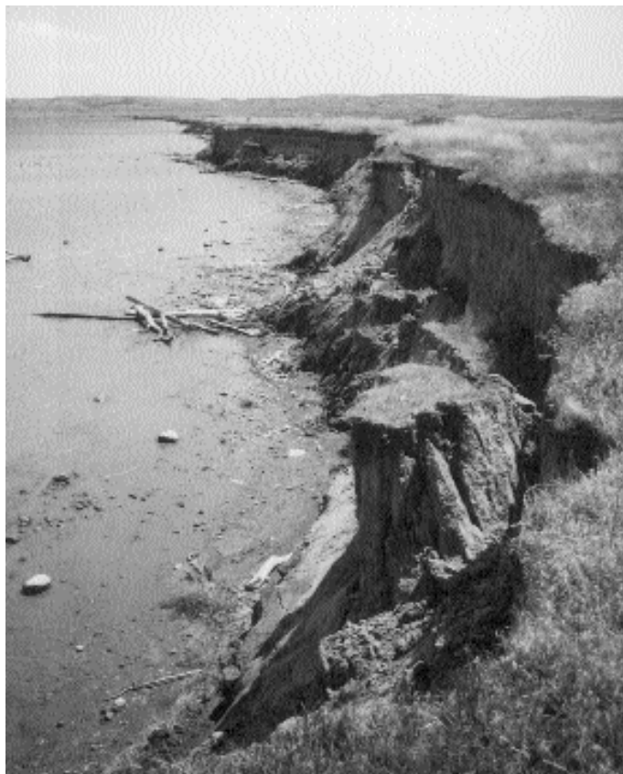
Severe erosion along the middle Missouri River (courtesy U.S. Army Corps of Engineers).
