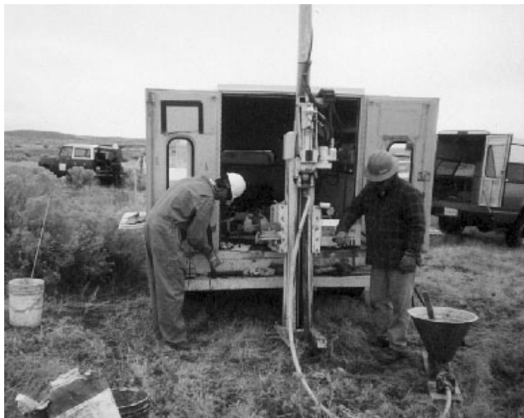
Technicians at the Hanford 100 Area 126-F-1 Ash Pit performing grouting operations with the Small-Diameter Geophysical Logging System.
