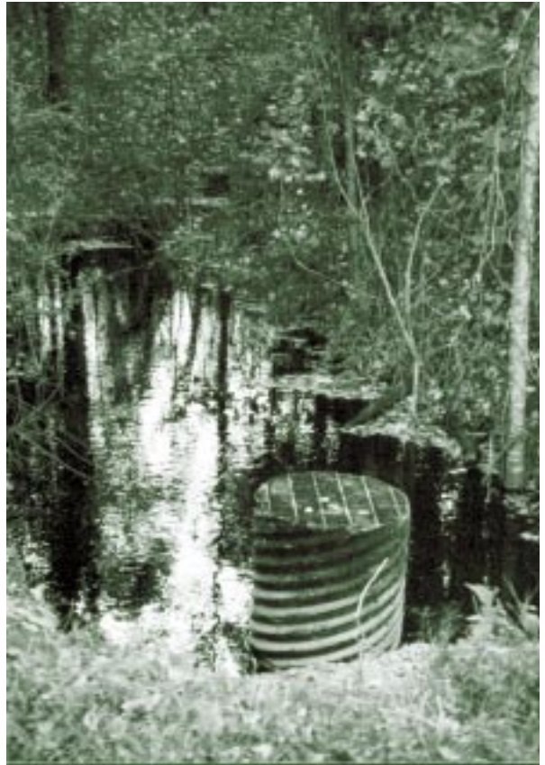
Wetland BMP—outfall pipe regulating water level in urban wetland system.
