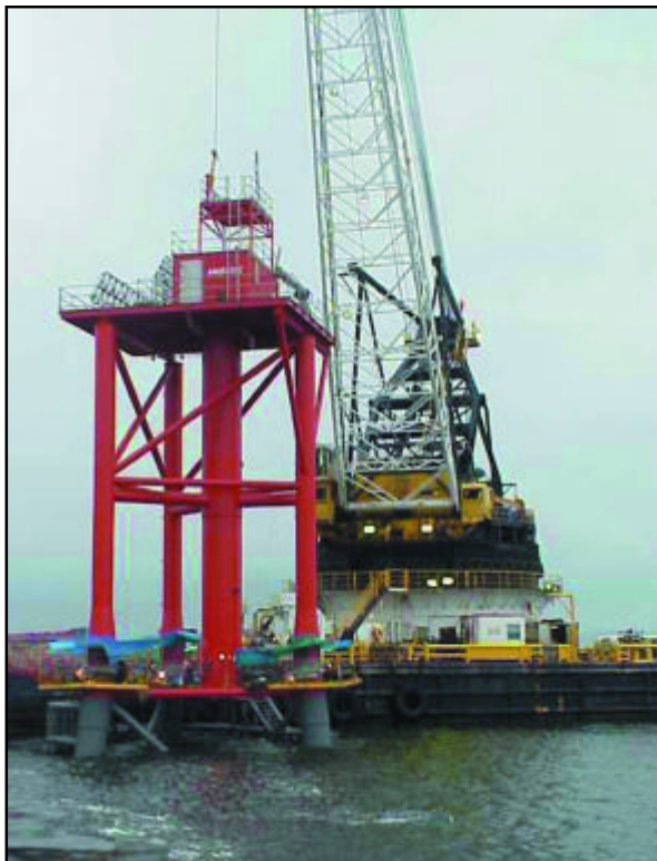
The Ambros Light, located 7.5 miles east of Sandy Hook, New Jersey, under construction. Ocean engineers are responsible for the design, construction and maintenance of Aids to Navigation.
