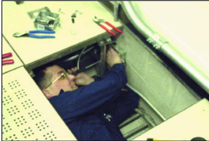
LT Al Yelvington, under access floor, installs an upgraded power distribution system for the Loran-C timing and control equipment at the Loran Support Unit, Wildwood, New Jersey. The LT is a 1992 graduate of Michigan Tech University with a Bachelor of Science degree in Scientific and Technical Communications.
