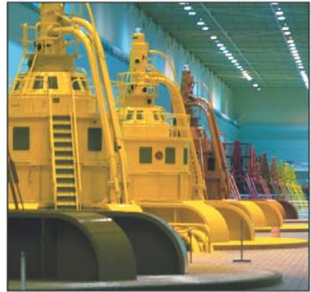
Generators at The Dalles Dam (OR)
