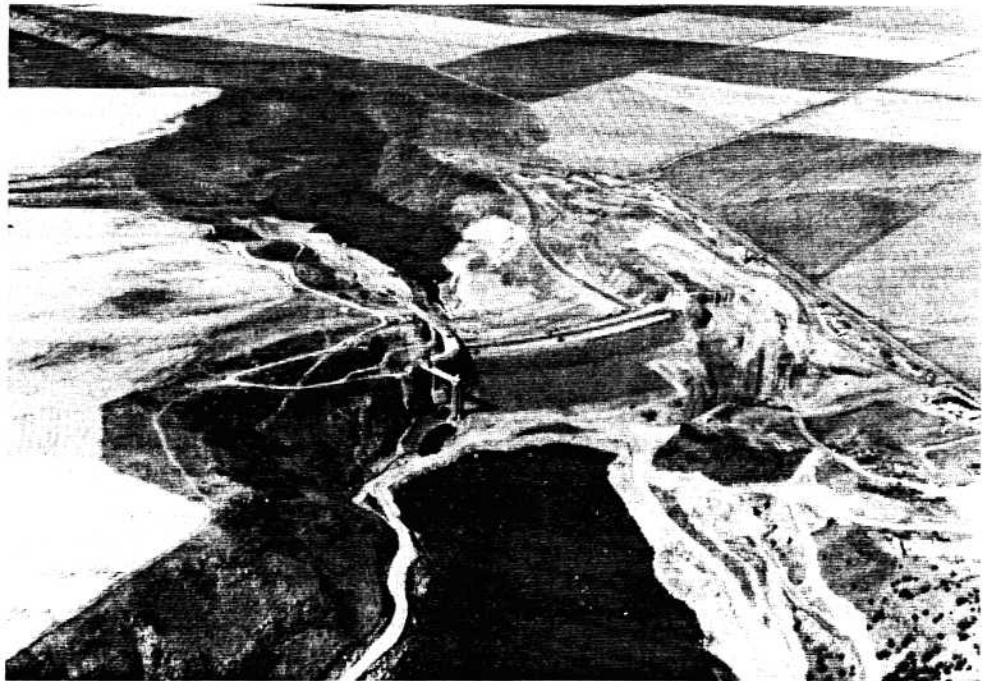
RIRIE DAM CONSTRUCTION - 1975 Spillway Channel at Right Abutment Outlet Works at Left Abutment
