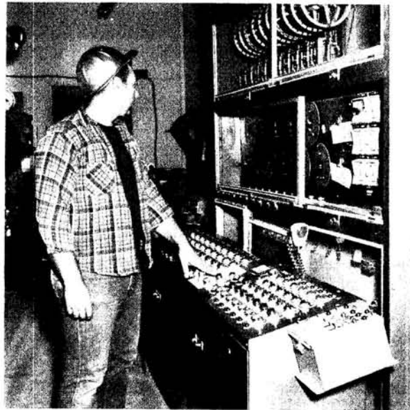
BATCH PLANT CONTROLS.
