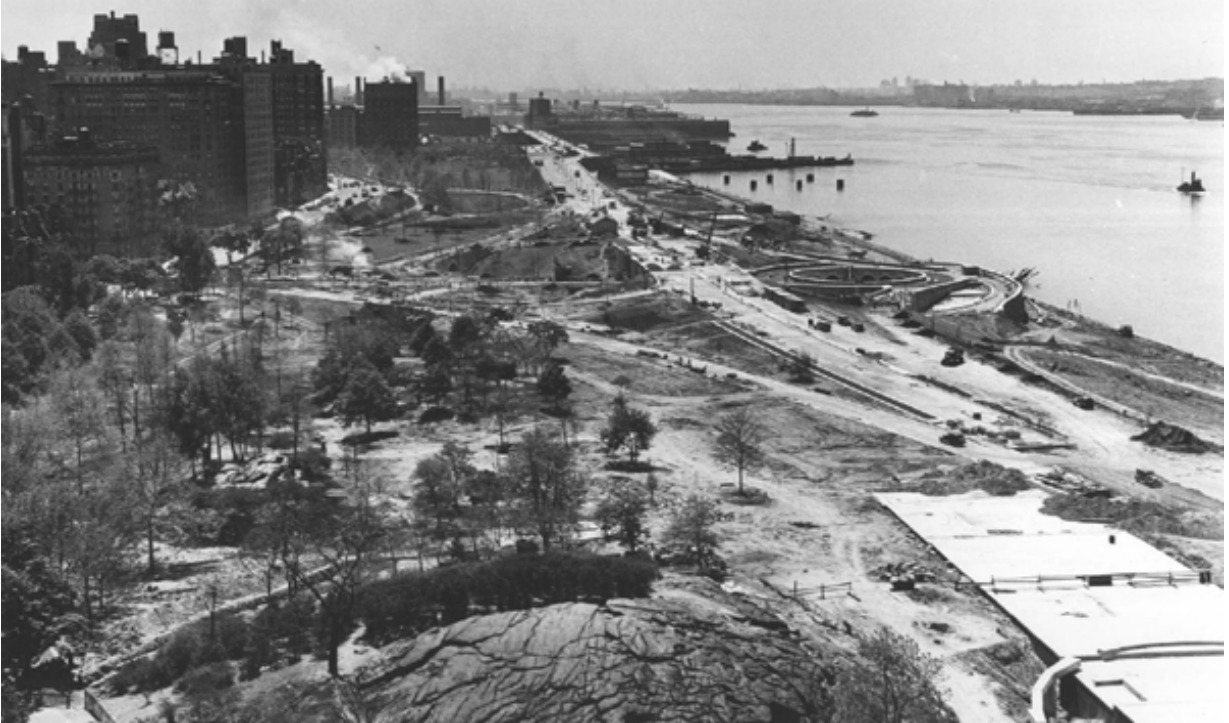
South-bound view from 79 th St. of the Henry Hudson Parkway under construction, circa 1936-37.
