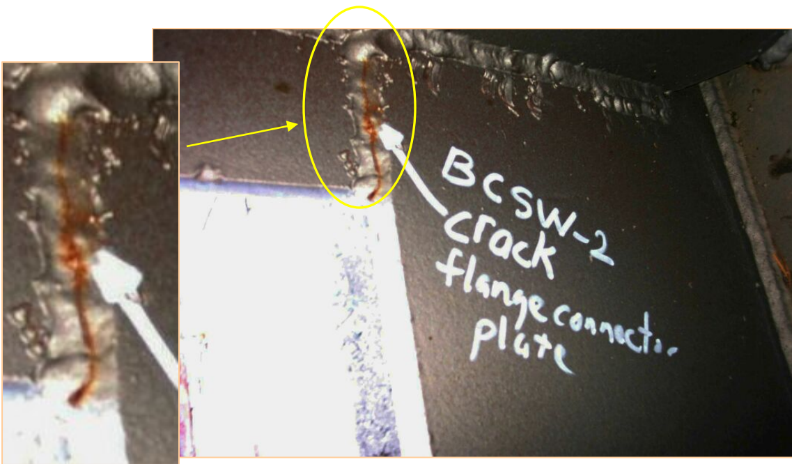
Crack at flange diaphragm plate
