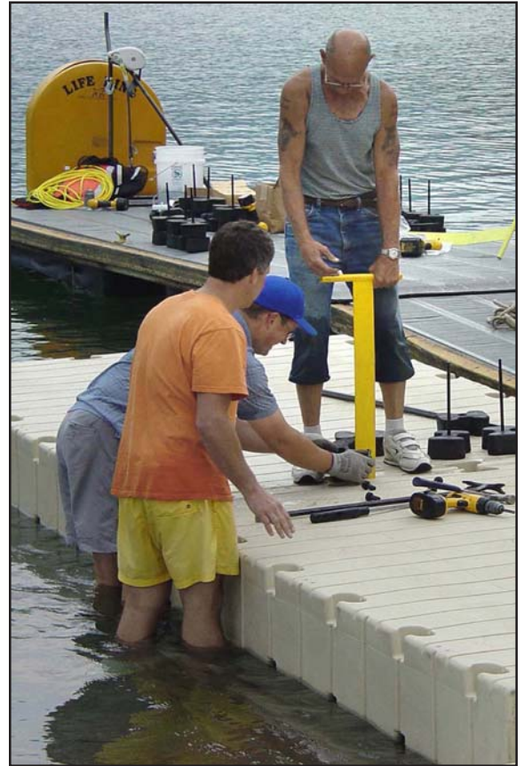
Right, Caleb Hall, a District family member (wearing the orange shirt), helps E-Z Dock representatives assemble dock sections for installation on Elk Creek.
