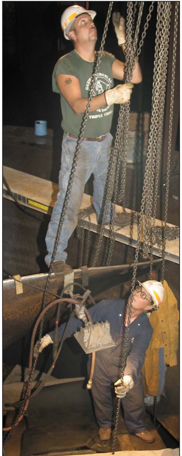
Above, Rich Johnson, utilityman, adjusts the chainfalls from above while Carey Basel, welder, monitors the position of the blade section as they suspend it and lock it in place for welding (photo by Gina Schwetz). Left, Carey Basel uses a peener to flatten and smooth-out a spot in the welding. Once workers got the broken section back into the scrollcase, it took only five weeks for them to reattach the blade, welding it from the top and bottom back onto the turbine (photo by Sam Liming).
