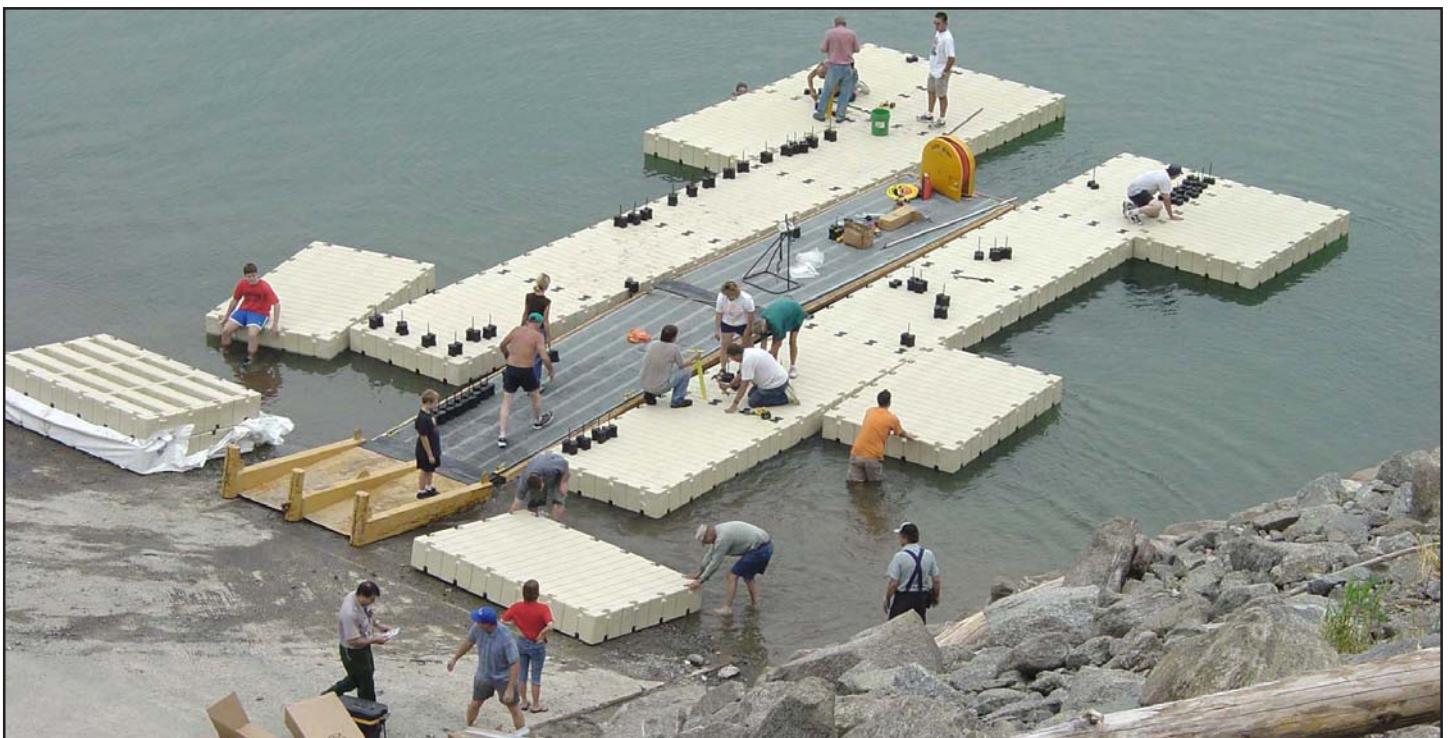
Volunteers, manufacturer representatives and Dworshak personnel, assemble the new docks at the Bruce's Eddy boat ramp.
