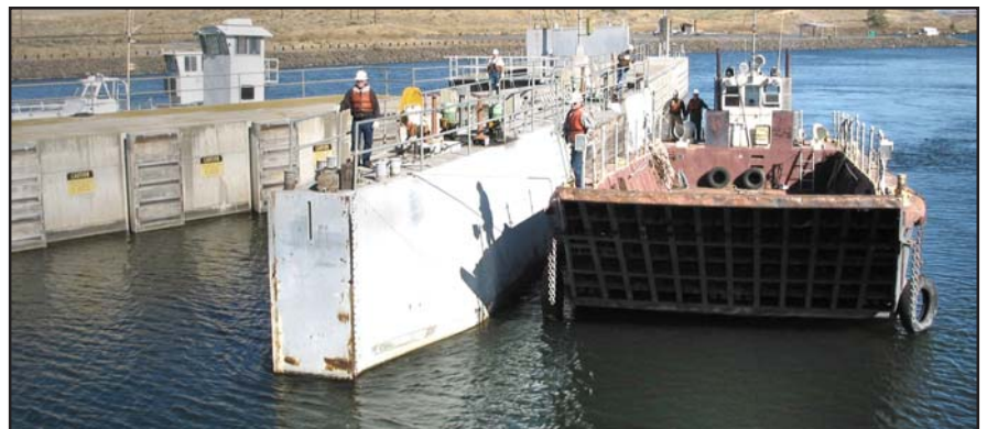
Above, Ice Harbor workers use a World War II landing craft to maneuver the bulkhead into the navigation lock. Left, Bill Rose and Marvin Cramer, get an up-close look at the damaged upstream gate as they are lowered into the lock to rescue two salmon stranded between the bulkhead and the gate.
