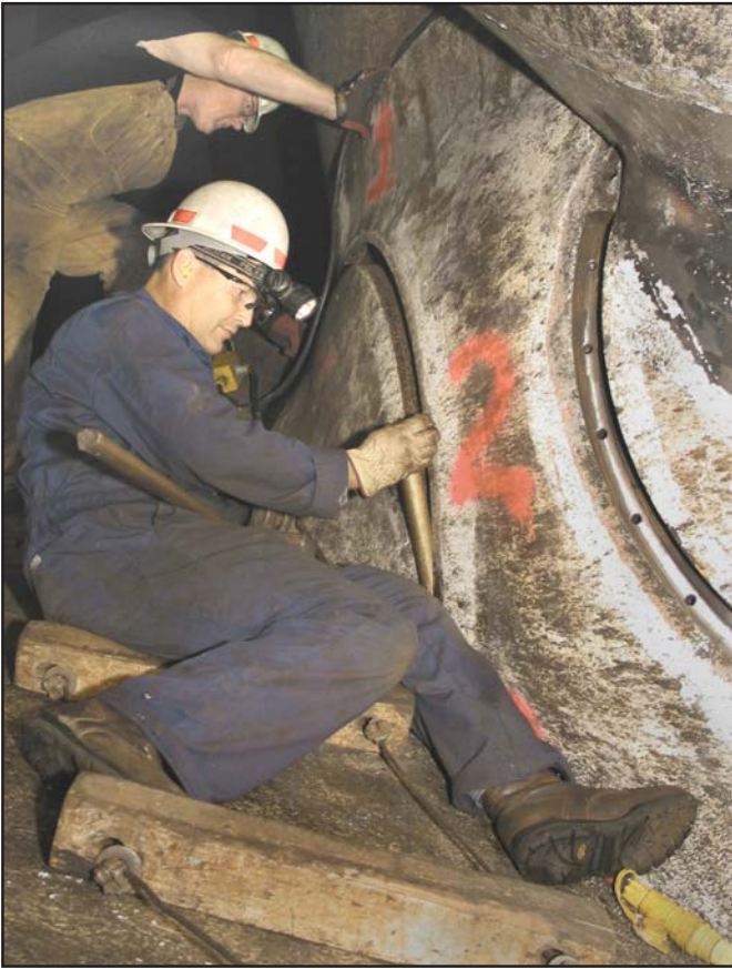
Clint LeMar, foreground, and Jim Allen, power plant mechanics at Lower Monumental Dam, remove the metal followers to access the old oil seals (photo by Gina Baltrusch).
