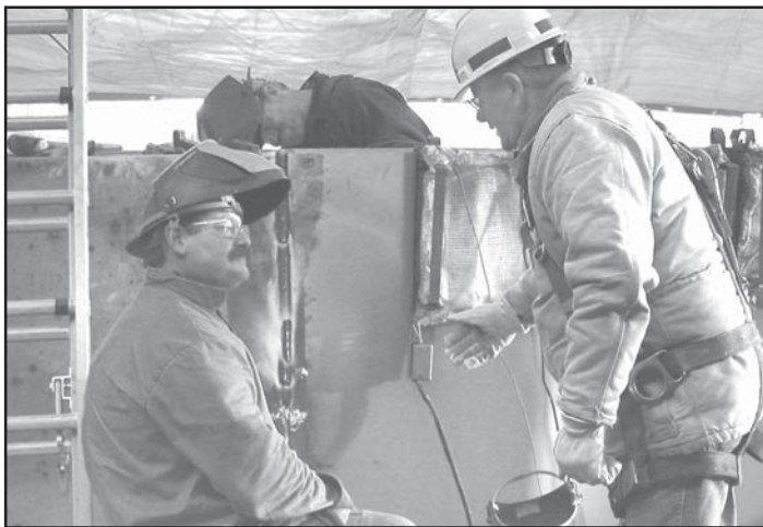
Gale Morgan (right), a quality assurance inspector in Walla Walla District's Construction Division, discusses the repair job with Ken Rader, a Dix Construction welder (photo by Gina Baltrusch).
