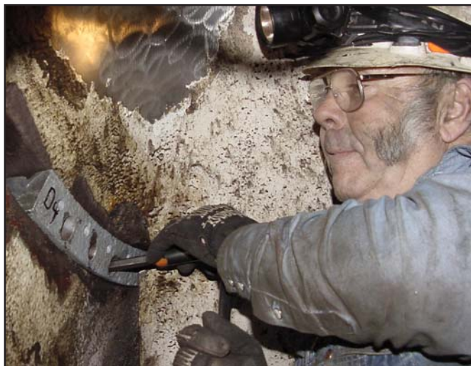
Leo Janes, power plant mechanic, loosens a bolt on a follower that workers need to remove to take out the old oil seals.(photo by Sue Walton).
