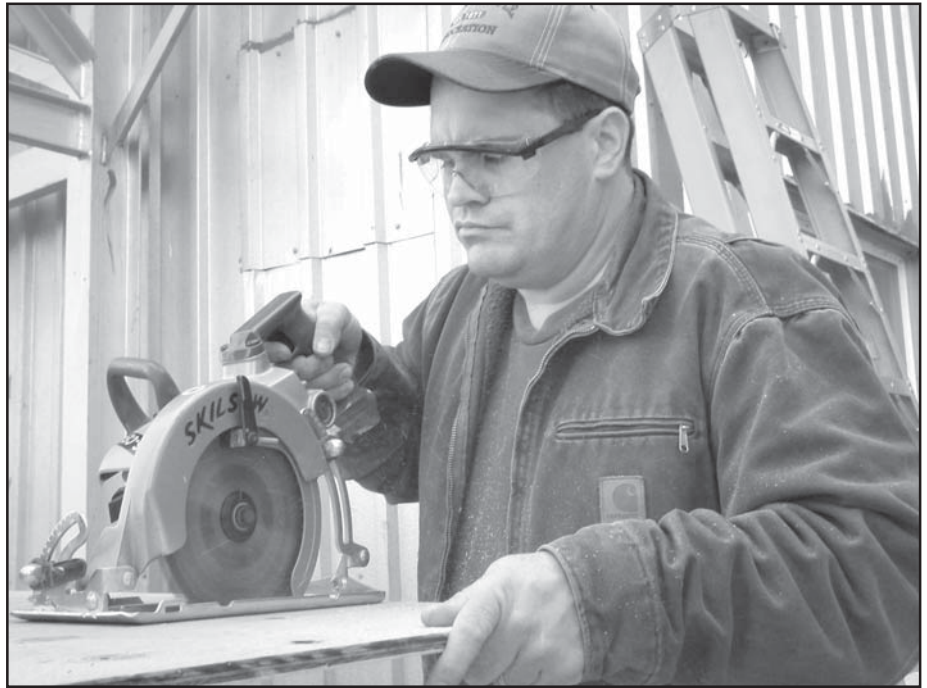
John Farthing, power plant trainee, saws a piece of plywood to panel an open area of the wall near the new training center's staircase.
