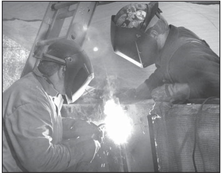
Ken Rader (left) and Troy White, Dix Construction welders, attach the new section into the navigation lock gate by welding it into place from both sides of the gate (photo by Gina Baltrusch).
