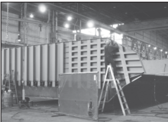
Above, workers at Thompson Metal Fabrication in Vancouver, Wash., build a new spillway weir for installation at Ice Harbor Dam on the lower Snake River. Right, Kevin Crum, a Walla Walla District project engineer and manager of the spillway weir project, explains to U.S. Army Corps of Engineers leaders and media representatives how the structure will function once in place.
