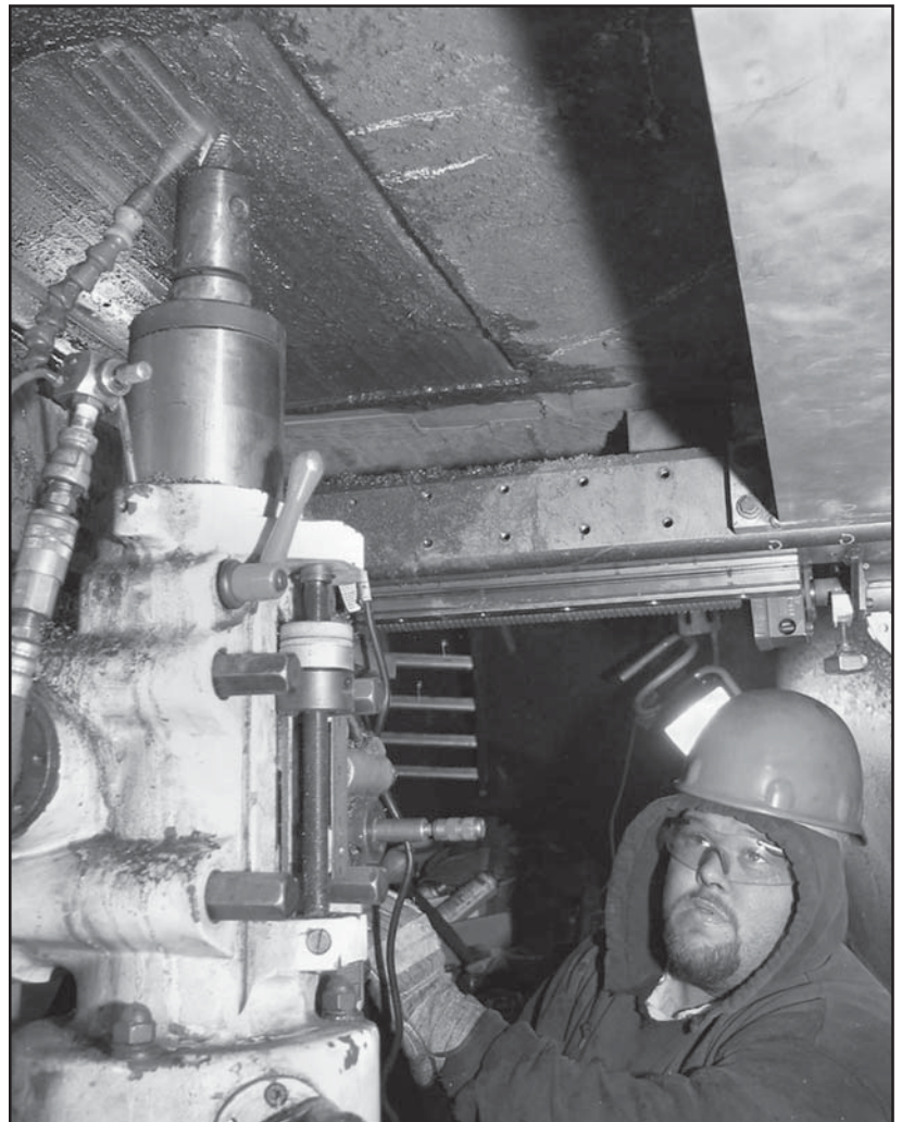
Kyle Kenoyer, welder, operates the portable milling machine to remove metal damaged by cavitation on one of the three turbines being repaired at Lower Granite Dam.
