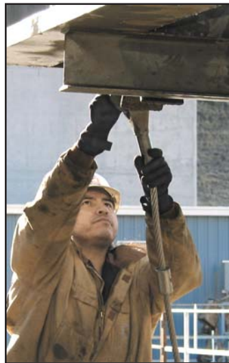
Tony Sijohn, power plant mechanic, disconnects a cable from the gantry crane's lifting beam after raising a turbine fish screen.
