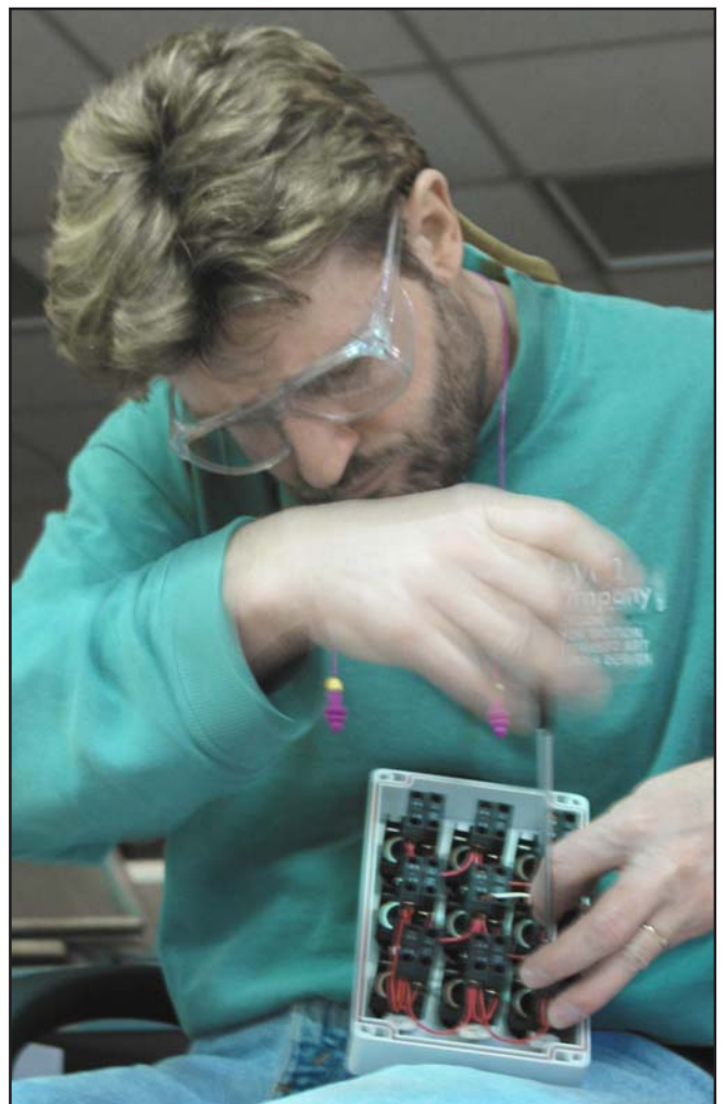
James Lyerly, power plant electrician, installs the wiring for one of the new push-button stations used for counting smolts at the dam's juvenile fish facility.
