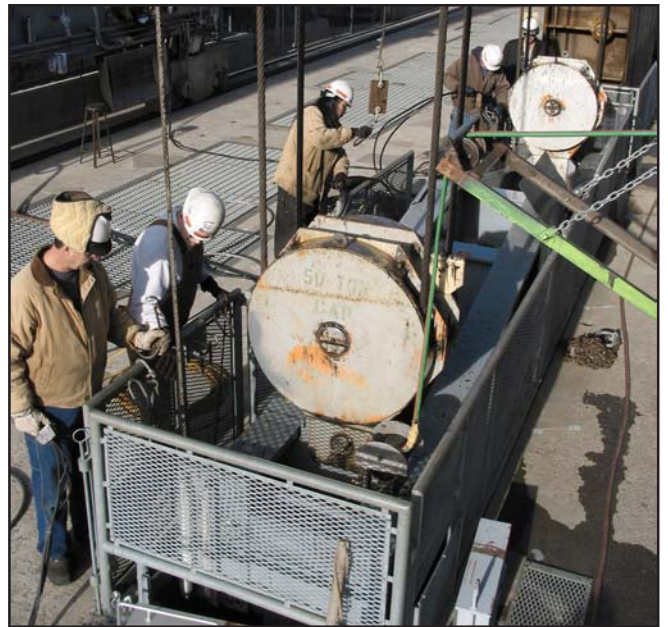
Power plant workers prepare to lock in place a turbine fish screen being raised by the dam's gantry crane for off-season cleaning and maintenance.
