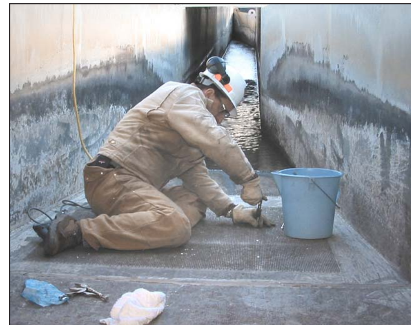
Rick Weis, biological technician, installs new, perforated, metal plates in the fishway leading to the separator to help release excess water.
