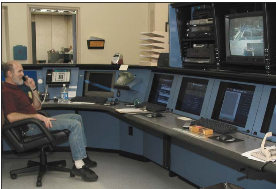
Above, Alan Schlachter, power plant shift operator, monitors the dam’s six generators from the control room. Right, Ed Baker, power plant mechanic, removes a main unit generator cooling water strainer for cleaning.
