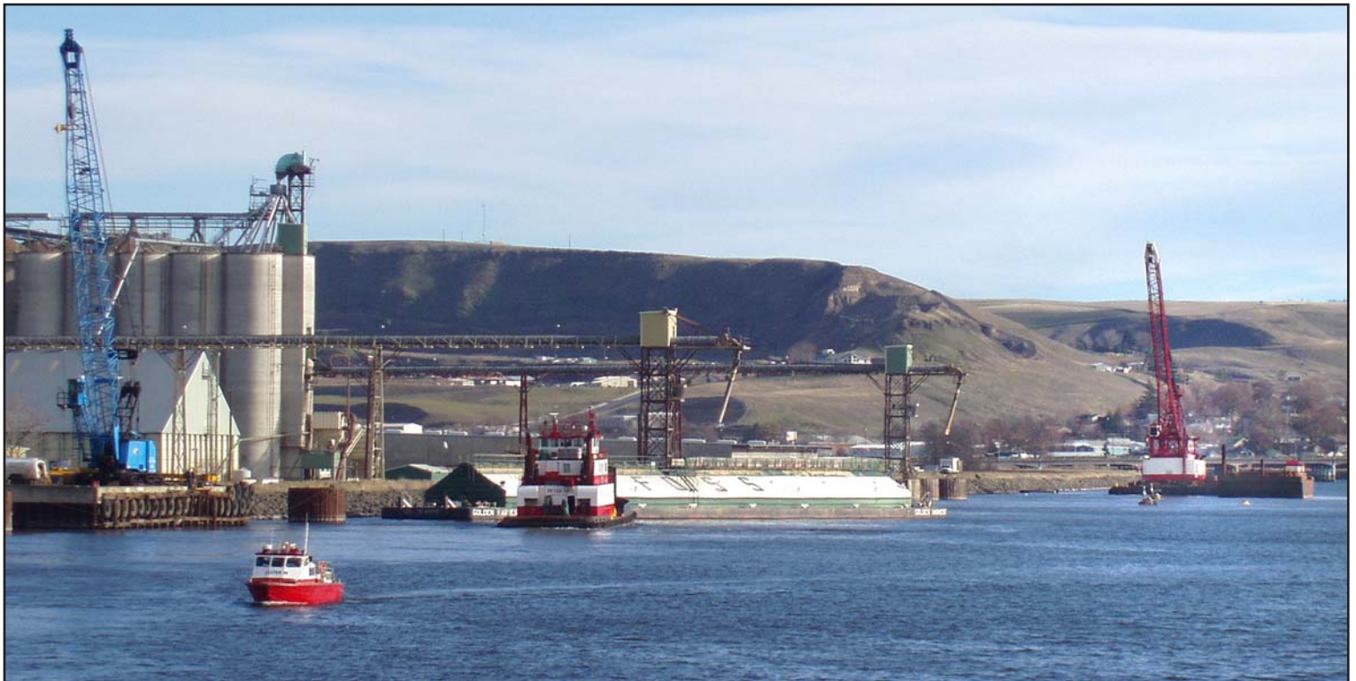
Photo provided by Manson Construction Company (taken by Kathleen Becker, MCC safety manger)
