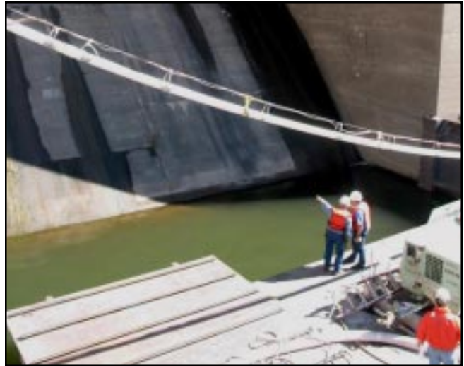
District project team members get an up-close look at construction progress below the spillway.
