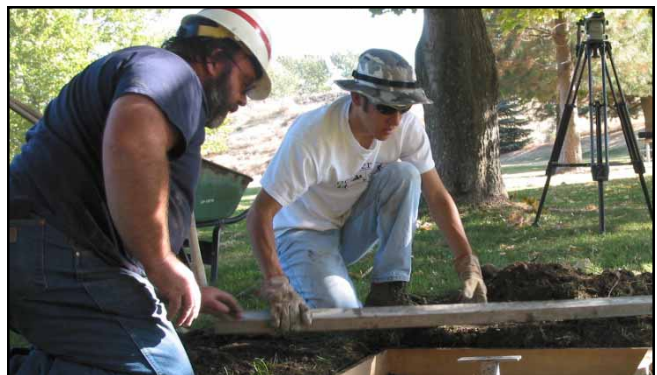
Dave Parker, Mill Creek maintenance worker, directs a student-volunteer as he digs out a form for concrete pads for new park benches and trash containers.
