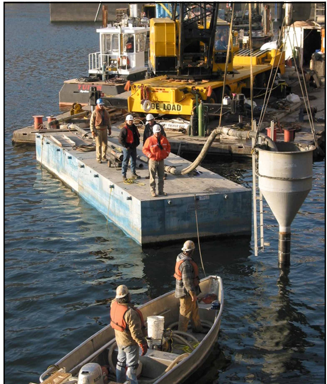
Steve Tatro, orange coat, a Walla Walla District concrete expert, inspects progress on the basin repair work done Nov. 26. Behind Tatro, wearing blue jeans and an orange safety vest, Steve Thompson, a Mill Creek park ranger and certified dive inspector, monitors diver activity at the repair site.
