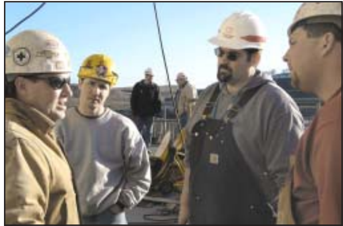
Brannon Schneider, Knight Construction, Brian Collier, Johns Electric, Inc., Jonathan Harrell, and Dave Donner, Knight Construction, discuss how to adjust performance of the butterfly valves.
