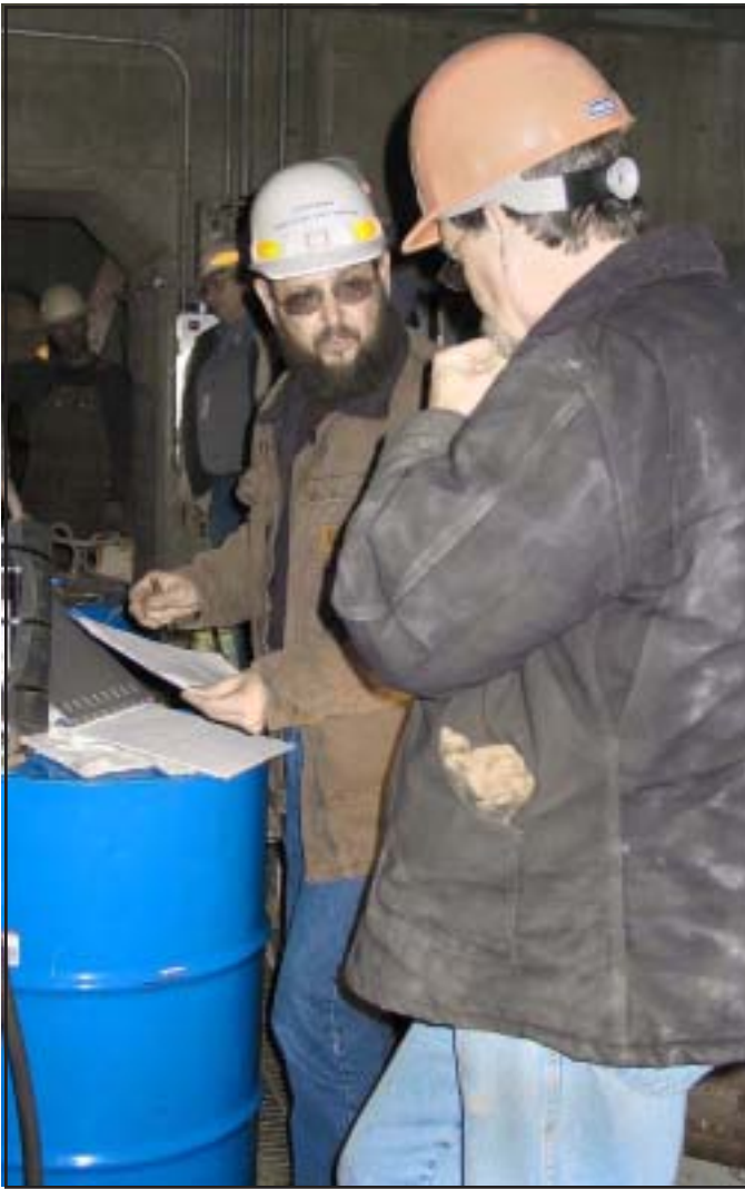
Lester Maier, power plant shift operator at Ice Harbor, and Butch Holt, McClure and Sons, Inc., project superintendent, assess how to proceed on adjustments to the new pumps.
