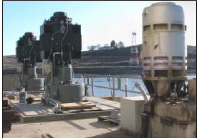
Two new impeller-type vertical pumps with 450-horsepower motors were tested and put into operation in late February.
