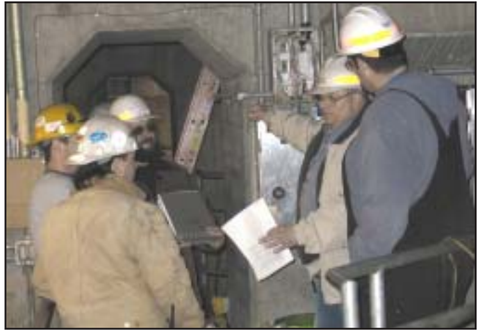
Co-op student Jonathan Harrell, far right, and Frank Scopa, project engineer, inside right, plan how to conduct a test of the new auxiliary water supply pumps with project contractors.
