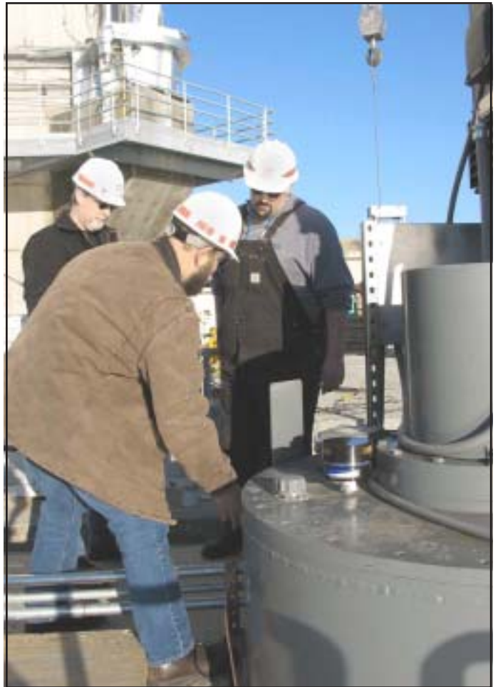
Jonathan Harrell, right, Construction Division co-op student, Scott Sutliff, left rear, Ice Harbor Lock and Dam operations manager, and Lester Maier, left front, power plant shift operator, inspects a new pump.
