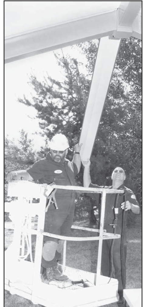
Dave Parker and Bob Radke, maintenance workers at Mill Creek Project, guide the final roofing piece on a picnic shelter at Bennington Lake.
