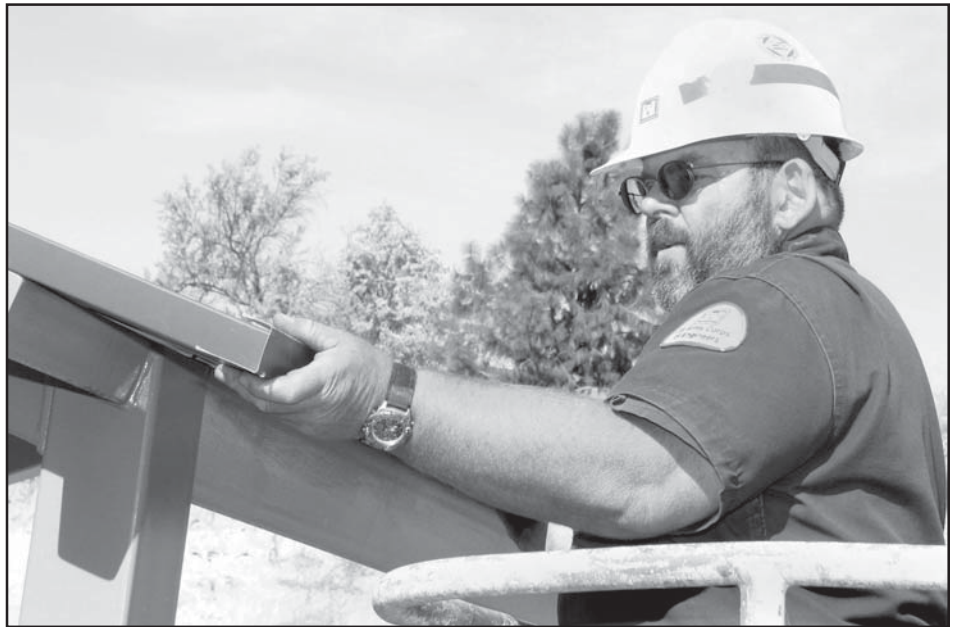
Dave Parker, maintenance worker, puts the roofing pieces on one of four new picnic shelters at Mill Creek Project’s Bennington Lake.
