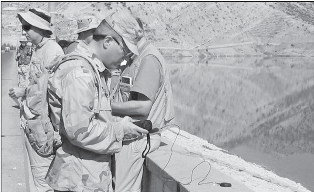
Deputy District Commander Maj. Harry Cunningham leads a dam assessment team as they evaluate the condition of the Dihok Project in Iraq. (U.S. Army Corps of Engineers photo)
