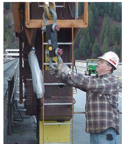
After unloading the gantry crane motors, Sonny Mitchell, a Dworshak utilityman, guides the shackles as a 20-ton boom truck lowers its hook
