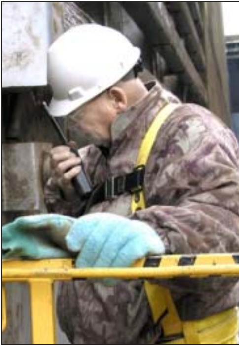
Gary Mellstrom, Lower Granite Dam's mechanical section foreman, climbs inside the manbasket and radios to crane operators on top of the navigation lock instructing them to hoist him up while he greases the gate seal.
