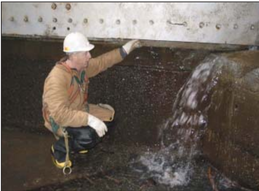
Bob Hollenbeck, the District's chief of structural design in Engineering Division, inspects the bottom of Lower Granite Lock's north gate door.
