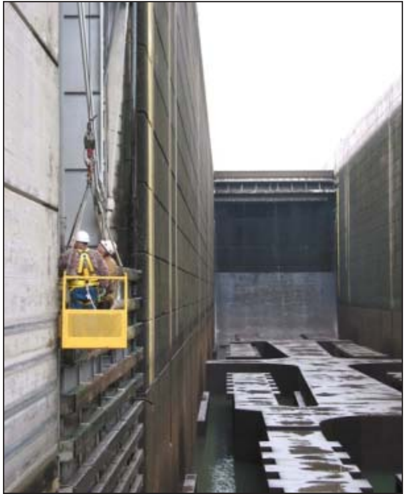
Bob Hollenbeck, chief of structural design for the District, and Gary Mellstrom examine the dry spots on the quoin seal.
