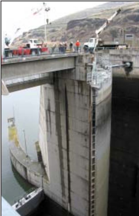
Lower Granite Lock and Dam maintenance and operations workers watch over the guardrail as lock operators test the gate to see if the waxy grease applied to the seals will fix the problem.
