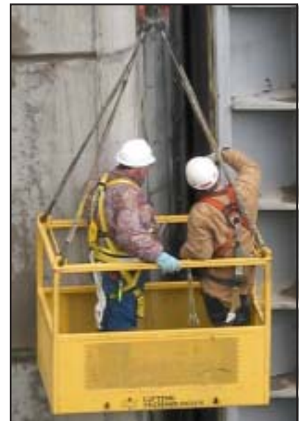
Gary Mellstrom and Bob Hollenbeck use a manbasket to inspect the 123-foot-high gate.
